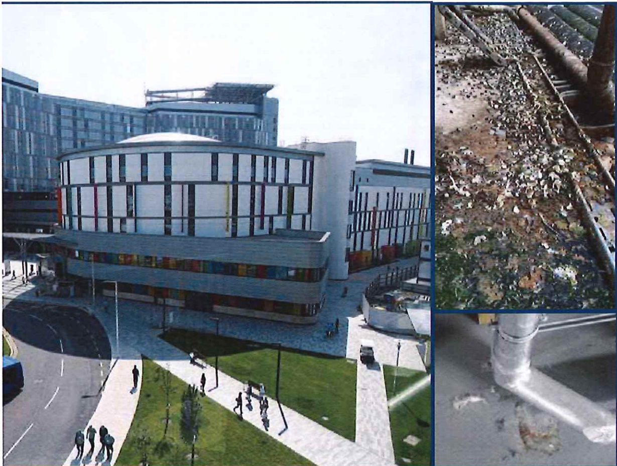
Outstanding repairs and the discovery of bird droppings have heightened infection fears at QEUH
