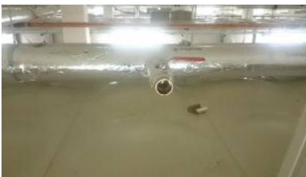
Emergency bypass points fitted around CWSTs (bulk CWST 2 pictured)
