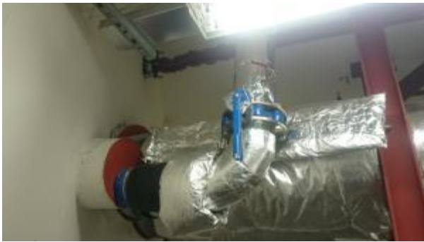
Govan Road mains entry point
