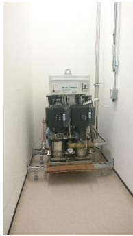
Dental Booster System (off at time of survey)
