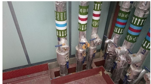
Tee-piece connections in risers.
