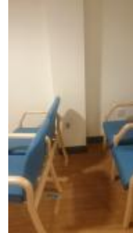
Unused equipment connection points found throughout building. These were not included in flushing regime at time of report.
