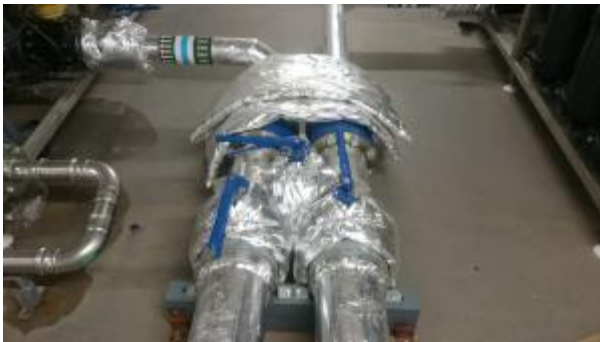
Filter set bypass/switch over point
