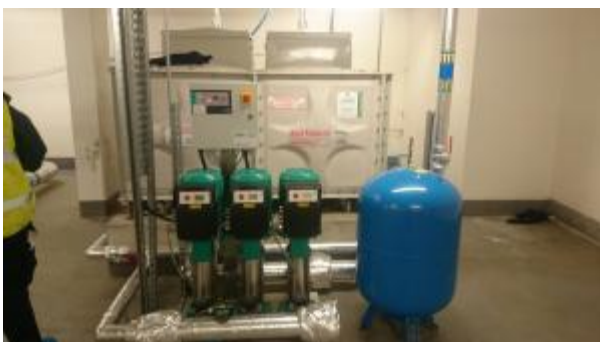
Trade boosters with manifold and expansion vessels (not flow through)
