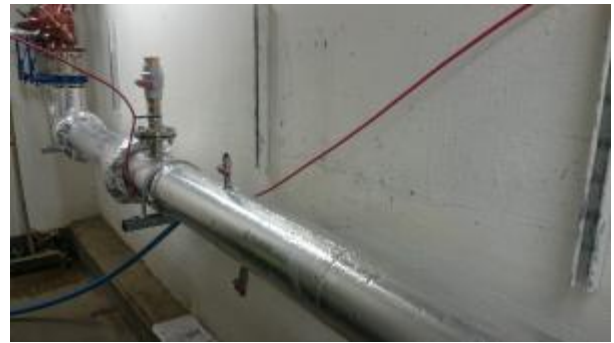
Govan Road mains – drain/injection points on supply to raw water CWSTs
