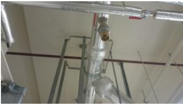
Typical emergency bypass connection point (Bulk CWST 1 pictured)
