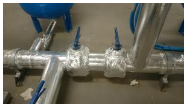
Bulk water pump bypass
