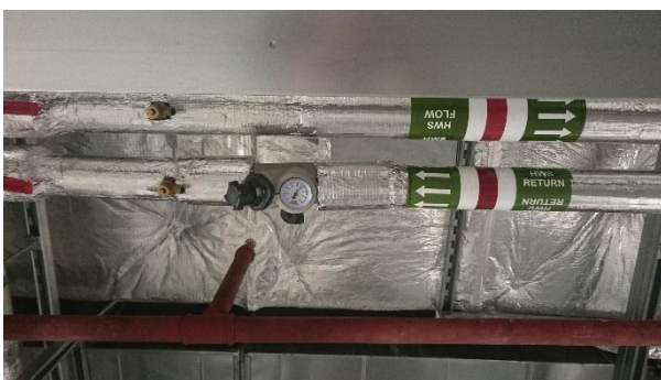
Low Hot return temperature (Gauge) Plantroom 33 (Cals 33-07/08/09 27/04/15)
