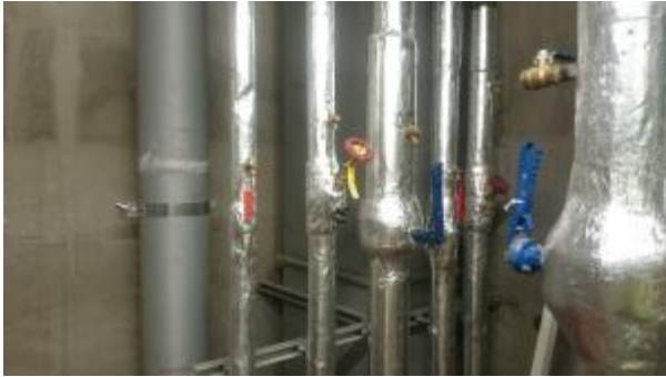
Generally drain points in risers appeared to be as close as possible to tee off point (New Childrens Hospital 4 th floor pictured)
