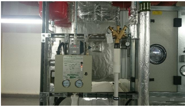
Runaround Coil Pressurisation Unit Connection (Plantroom 22)
