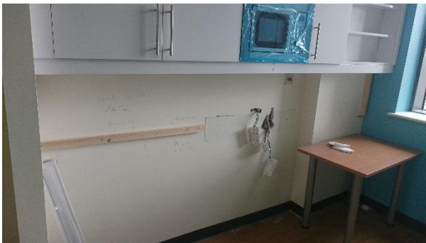
“Classroom” (Sch-077) still under construction – sink locations etc. marked on wall though no pipework fitted at time of survey.
