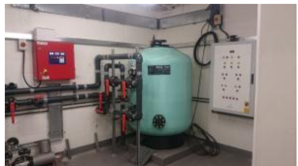
Hydrotherapy pool plant not yet completed or connected to water system at time of survey
