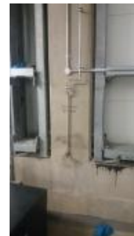
Typical bib tap from trade water system
