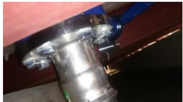
Typical CWST drain – tight to base
