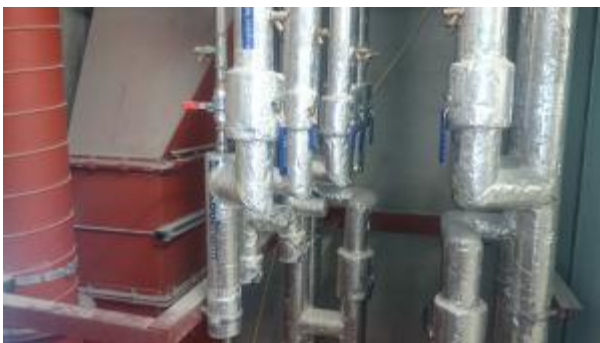
Drain points at bottom of risers/drops
