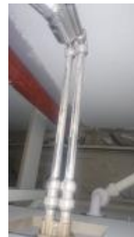
Some very local lengths of insulation missing
