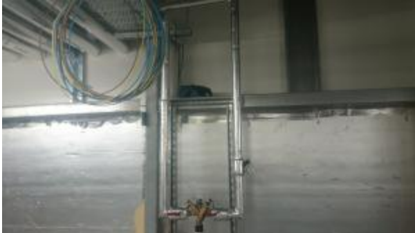
RPZ valve fitted on line to adiabatic chillers for MRI system. Check valve recommended at tee-off to all closed system tops or similar low flow areas to minimise potential for system contamination from low flow area.
