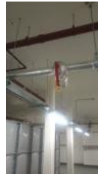
Sprinkler tank shut off at time of survey
