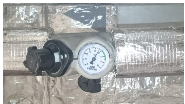
Low Hot return temperature (Gauge) Plantroom 33 (Cals 33-07/08/09 27/04/15)
