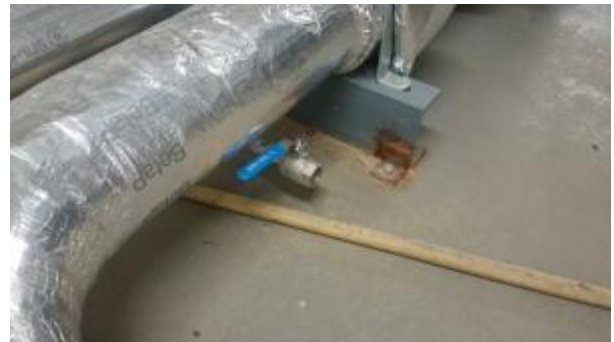
Drain off point at filter set
