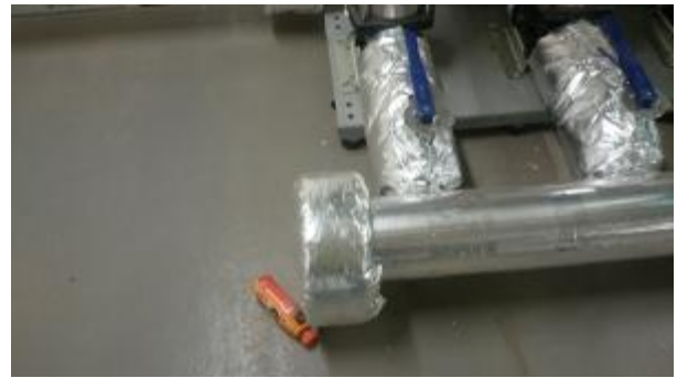
Typical pump manifolds (Bulk pumps pictured)
