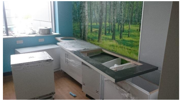
“Classroom” (Sch-077) still under construction – sink locations etc. marked on wall though no pipework fitted at time of survey.
