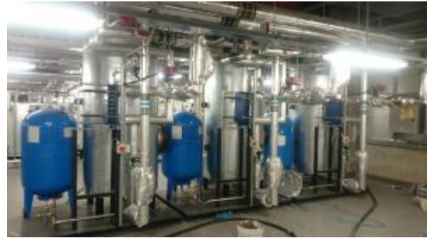
Typical calorifier set up. Expansion vessels are not flow through. (P31 04-05-06 pictured)
