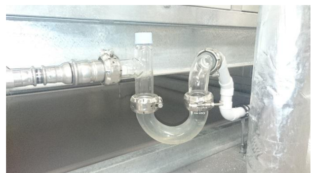
AHU Trap (Cloudy water within trap)
