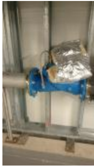
Flexible hoses on pressure reducing valves (assume to be EPDM)
