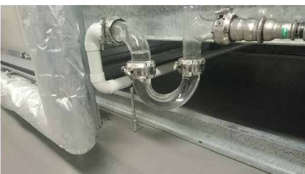
AHU Trap (Clear water within trap)
