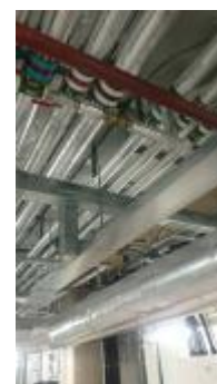
Non return valve on tee off to pressurisation unit/fast fill (P21 pictured)
