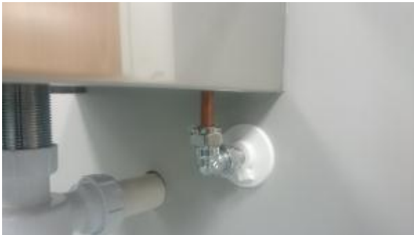
Small copper tails visible on Infra Red taps and Armitage Shanks taps in Endoscopy Wash Room
