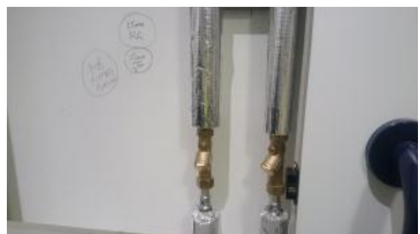
Angle strainer valves on supplies to TMV Taps (C1 23HU-047 pictured)
