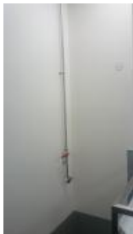
Unused equipment connection points found throughout building. These were not included in flushing regime at time of report.
