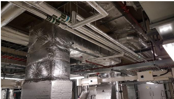
P31 Lines to Press Units (at Cals 01-02-03) (3)
