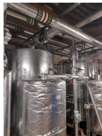
Plant Room 22 Offline Calorifier 1 (Mid)
