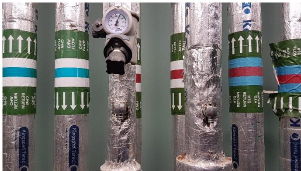
Typical Drain Cock in Riser (2)
