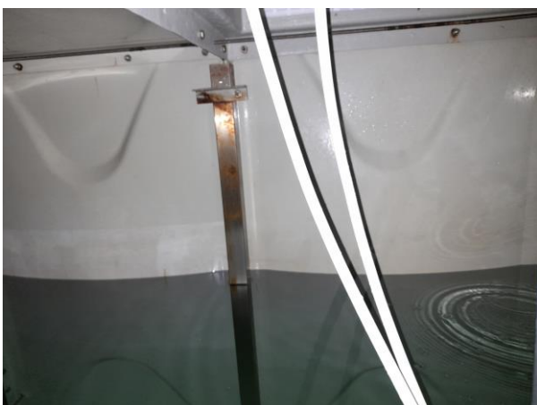
Example 2 of Corroded Internal Supports & Fittings in Filtered Water CWSTs
