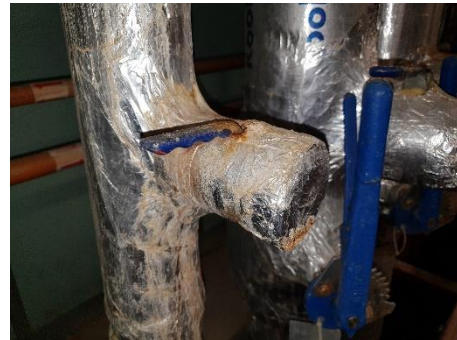
GENW15-068 Evidence of Leak (3)
