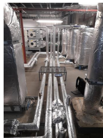
Plant Room 41 - Calorifiers 1-3
