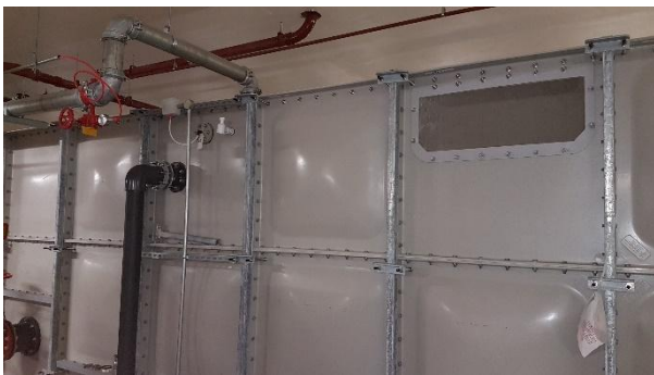
Basement Fire Tank Overflow
