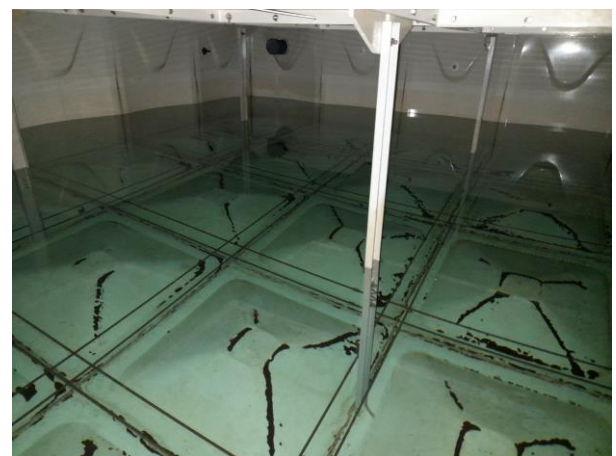
Raw Water CWST 1B Internal
