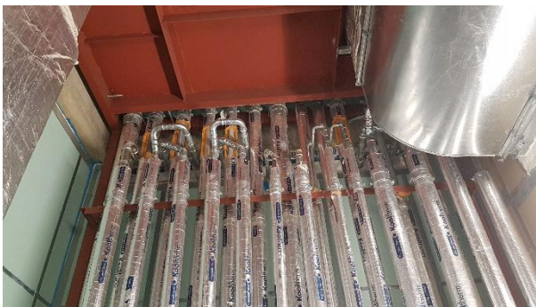
STW-012 Missing Insulation
