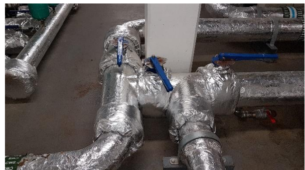
Basement Post Filter Pipework Link
