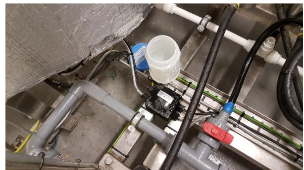
Endoscopy Wash Plant Leak
