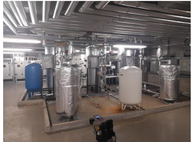
Plant Room 31 - Calorifiers 4-6
