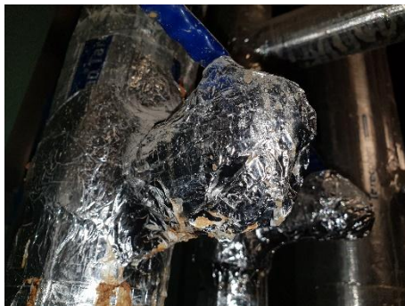
GENW16-068 Injection Point
