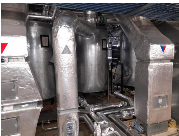
Plant Room 41 - Calorifiers 1-3
