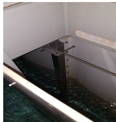
Raw Water Tank – Hollow S/S flange Support
