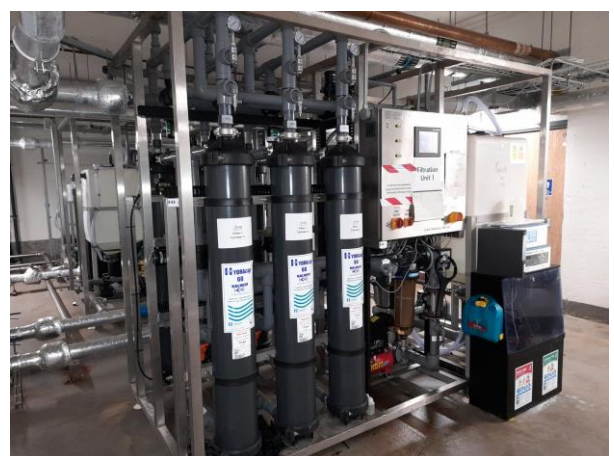
Raw Water CWSTs Filtration Unit 1
