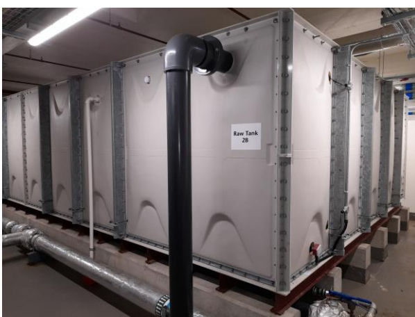
Raw Water CWST 2B
