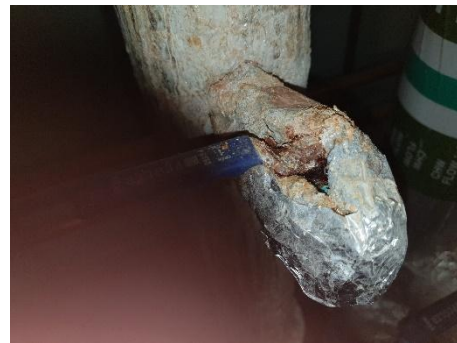
GENW19-068 Evidence of Leak (1)
