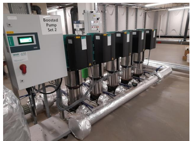
Filtered Water Booster Set 2
