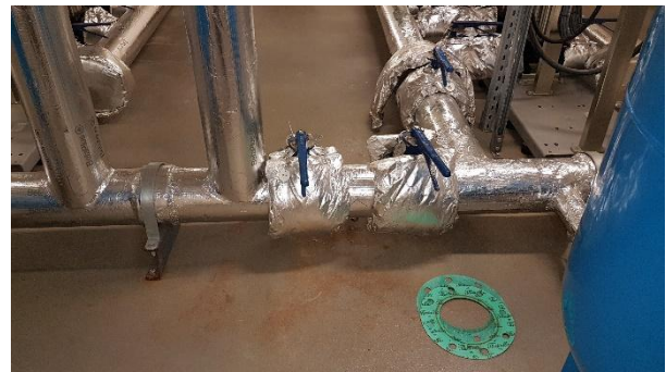
Basement Link Pipework between Pump Sets
