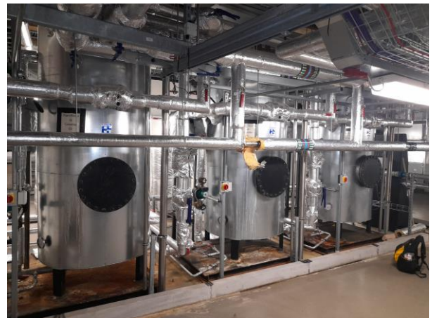
Plant Room 32 - Calorifiers 1-3
