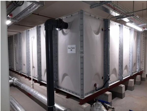
Raw Water CWST 1B
