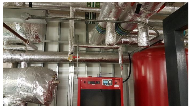
P31 Lines to Press Units (at Cals 01-02-03) (2)
