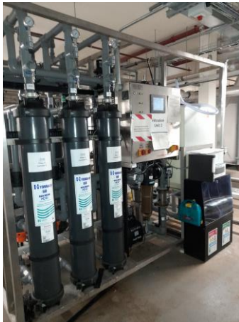
Raw Water CWSTs Filtration Unit 2
