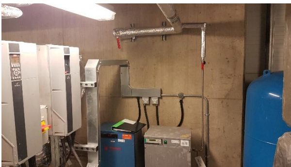
P31 Lines to Press Units (at Cals 01-02-03) (1)
