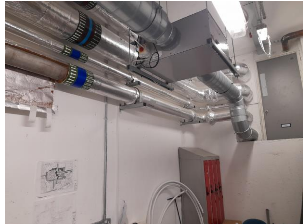
Hardgate Road Incoming Town Mains & Fire Tanks Main
