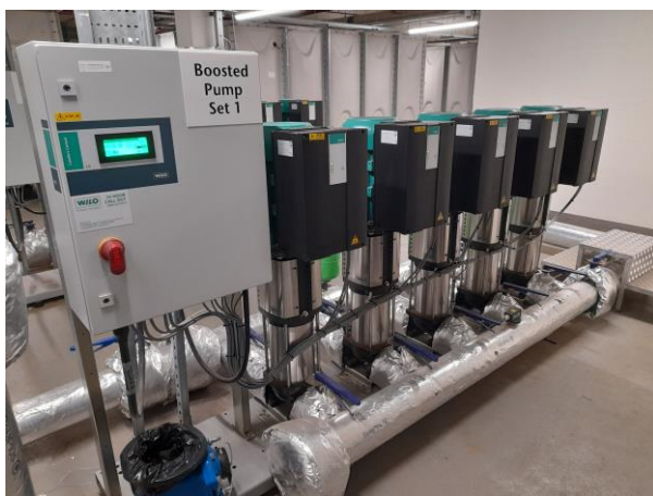
Filtered Water Booster Set 1
