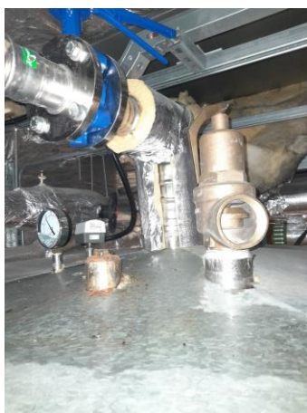
Open Face Safety Valve in Calorifier Plant Room 41
