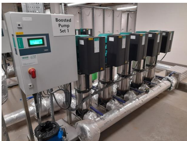
Filtered Water Booster Set 1
