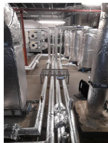
Plant Room 41 - Calorifiers 1-3
