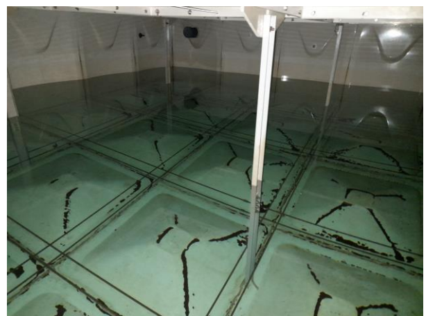
Raw Water CWST 1B Internal
