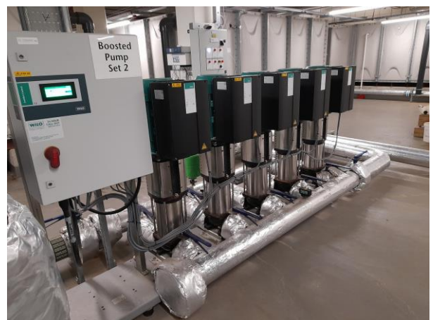
Filtered Water Booster Set 2
