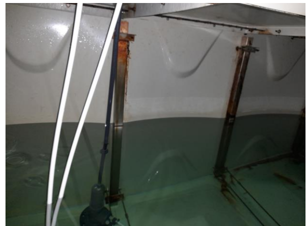
Example 1 of Corroded Internal Supports & Fittings in Filtered Water CWSTs
