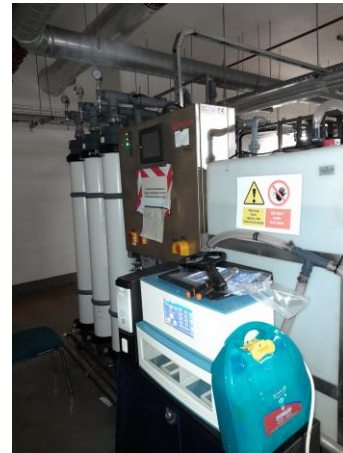
Raw Water CWSTs Filtration Unit 3
