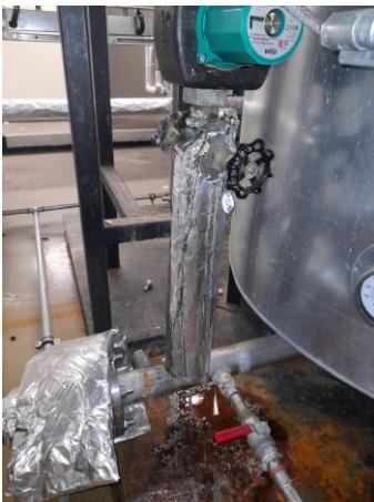
Plant Room 31 - Calorifiers 4-6
