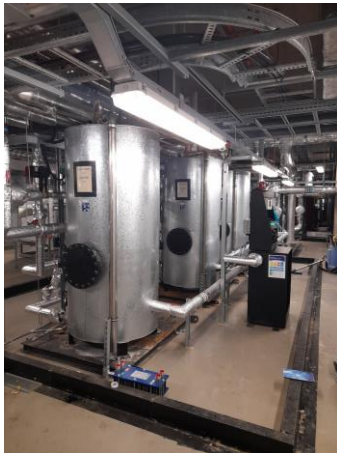
Plant Room 31 - Calorifiers 1-3
