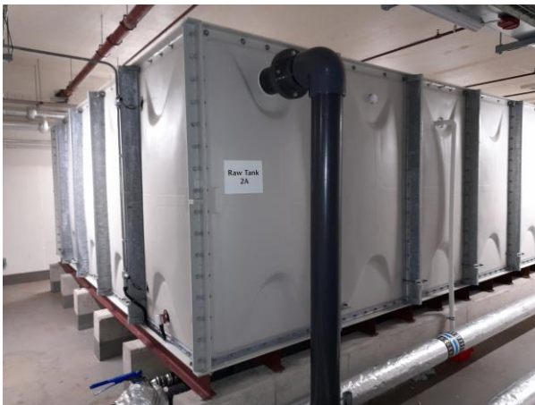
Raw Water CWST 2A
