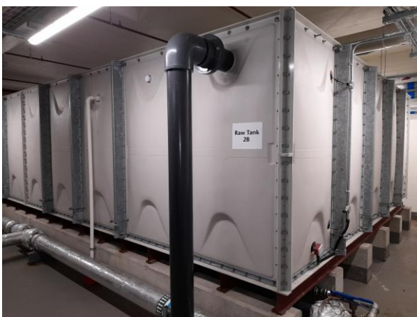
Raw Water CWST 2B
