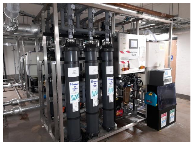
Raw Water CWSTs Filtration Unit 1
