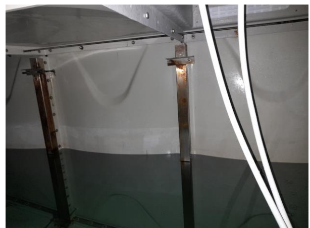
Example 3 of Corroded Internal Supports & Fittings in Filtered Water CWSTs
