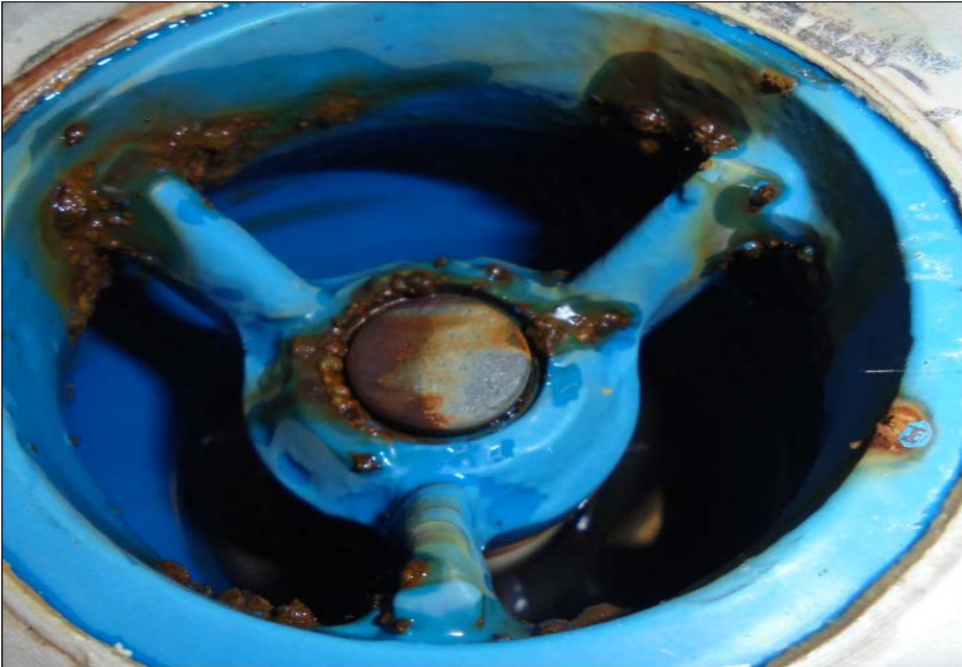
Fig 3 PR22 NRV HWS Return Line (internal)
