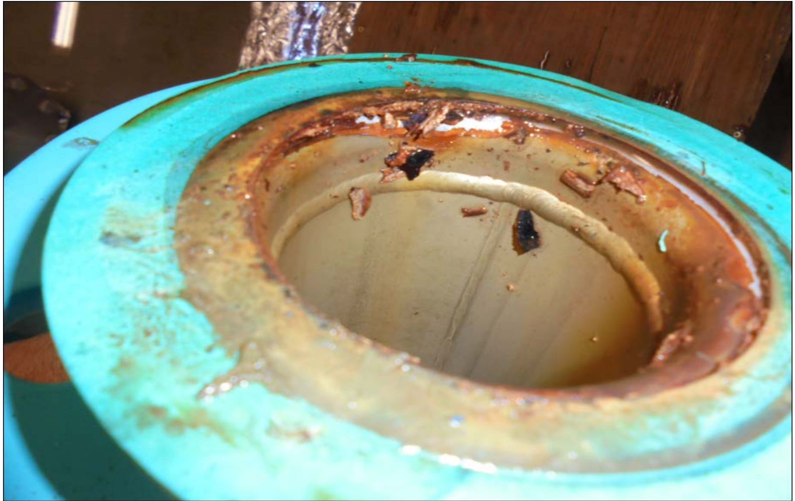
Fig 5 Booster Set 2 (Pump number 5 SS spool piece) (Source NHS Scotland)
