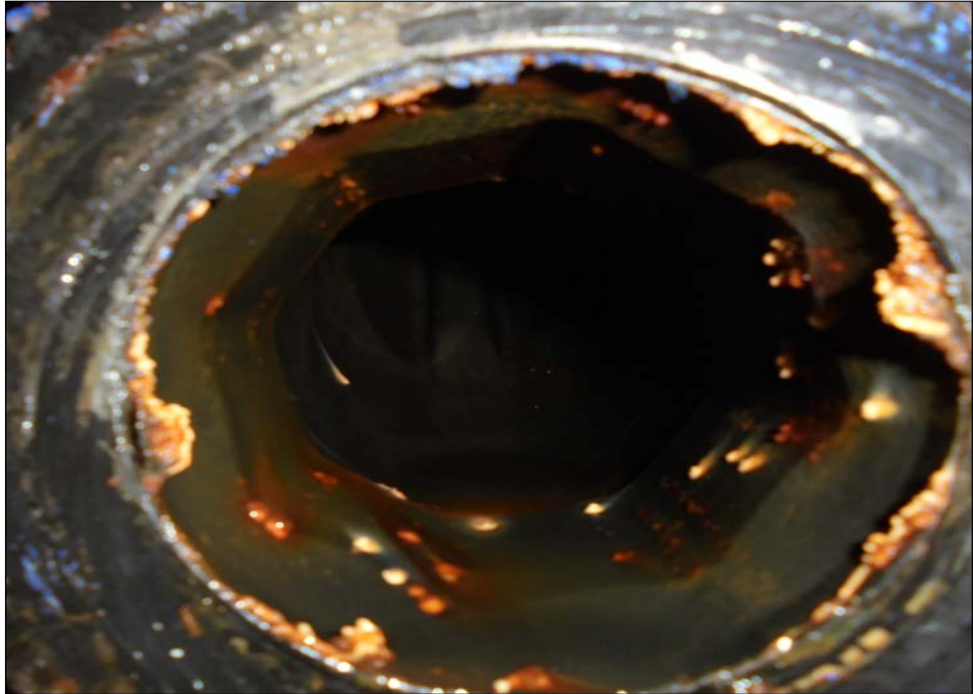
Fig 3 Booster Set 2 (Pump number 5) (Source NHS Scotland)
