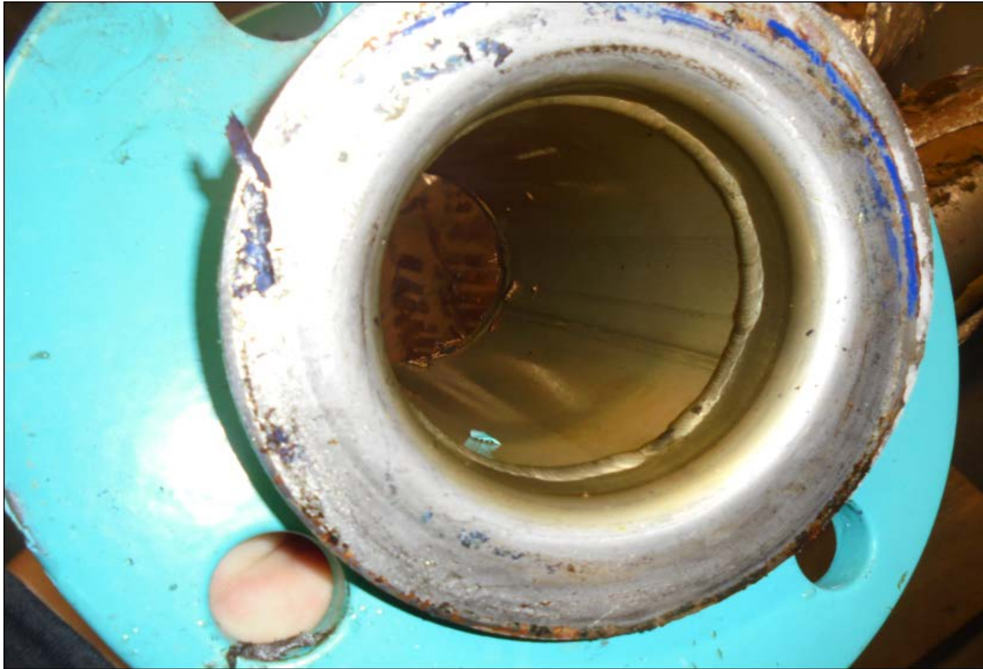
Fig 4 Booster Set 2 (Pump number 5 SS spool piece) (Source NHS Scotland)
