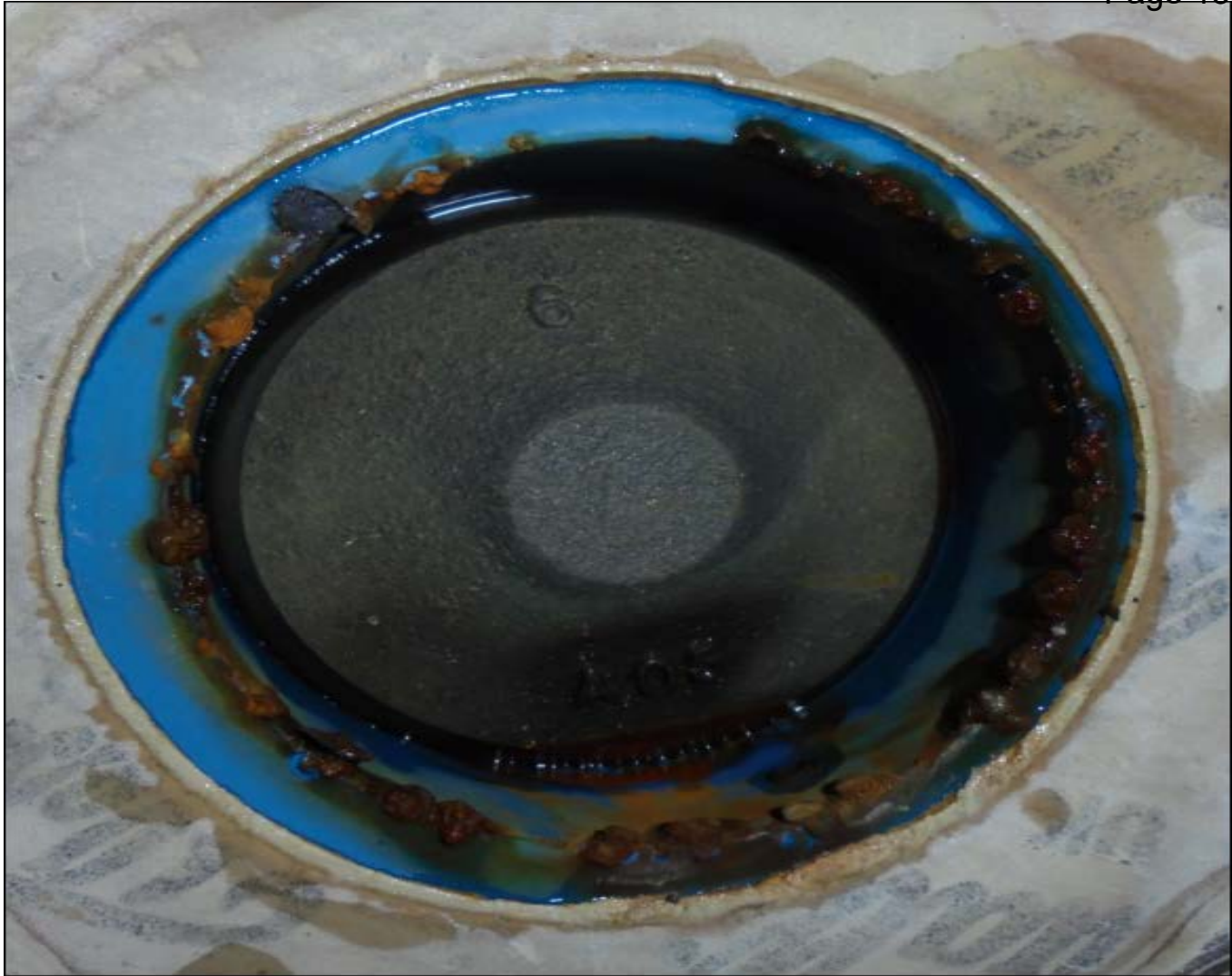
Fig 4 PR22 NRV HWS Return Line (internal)
