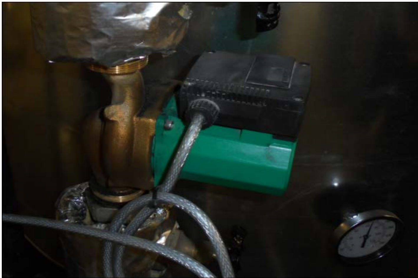
Fig 1 21Cal03 Shunt Pump
