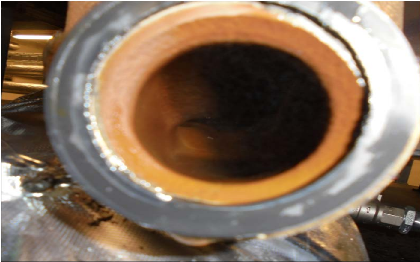
Fig 2 21Cal03 Shunt Pump (internal)
