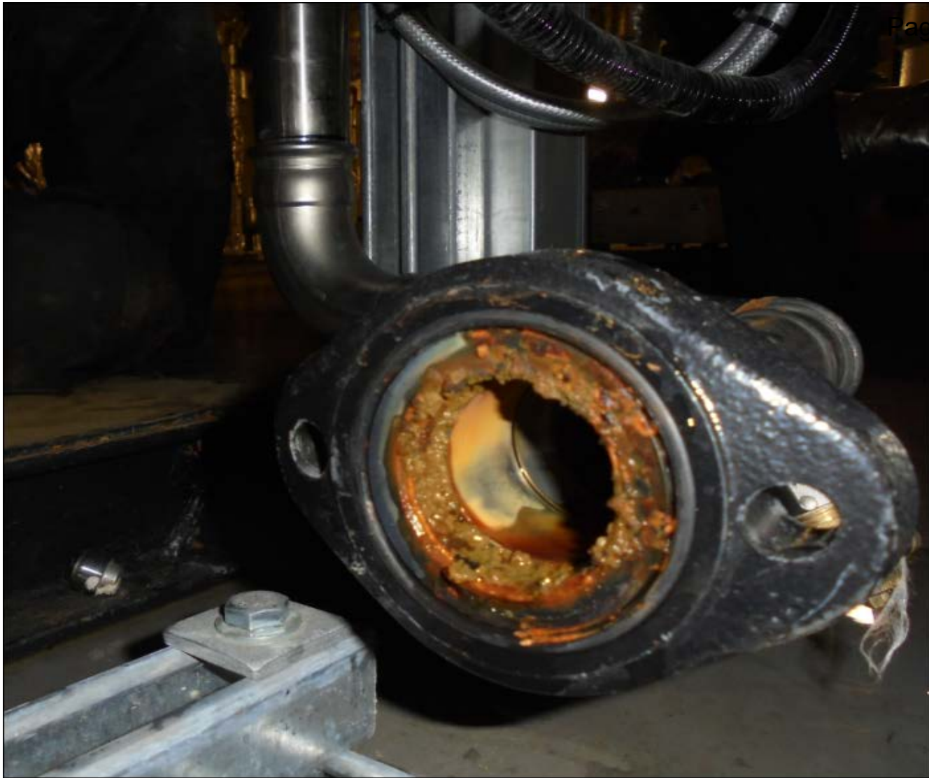
Fig 4 316L, 1, 2 and 3 HWS Return Pump (connections)
