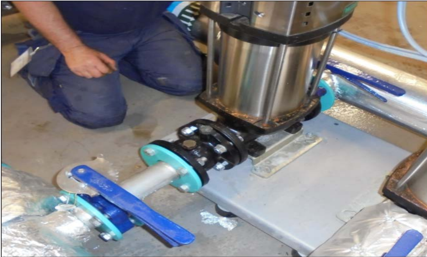
Fig 1 Booster Set 2 (Pump number 5) (Source NHS Scotland)
