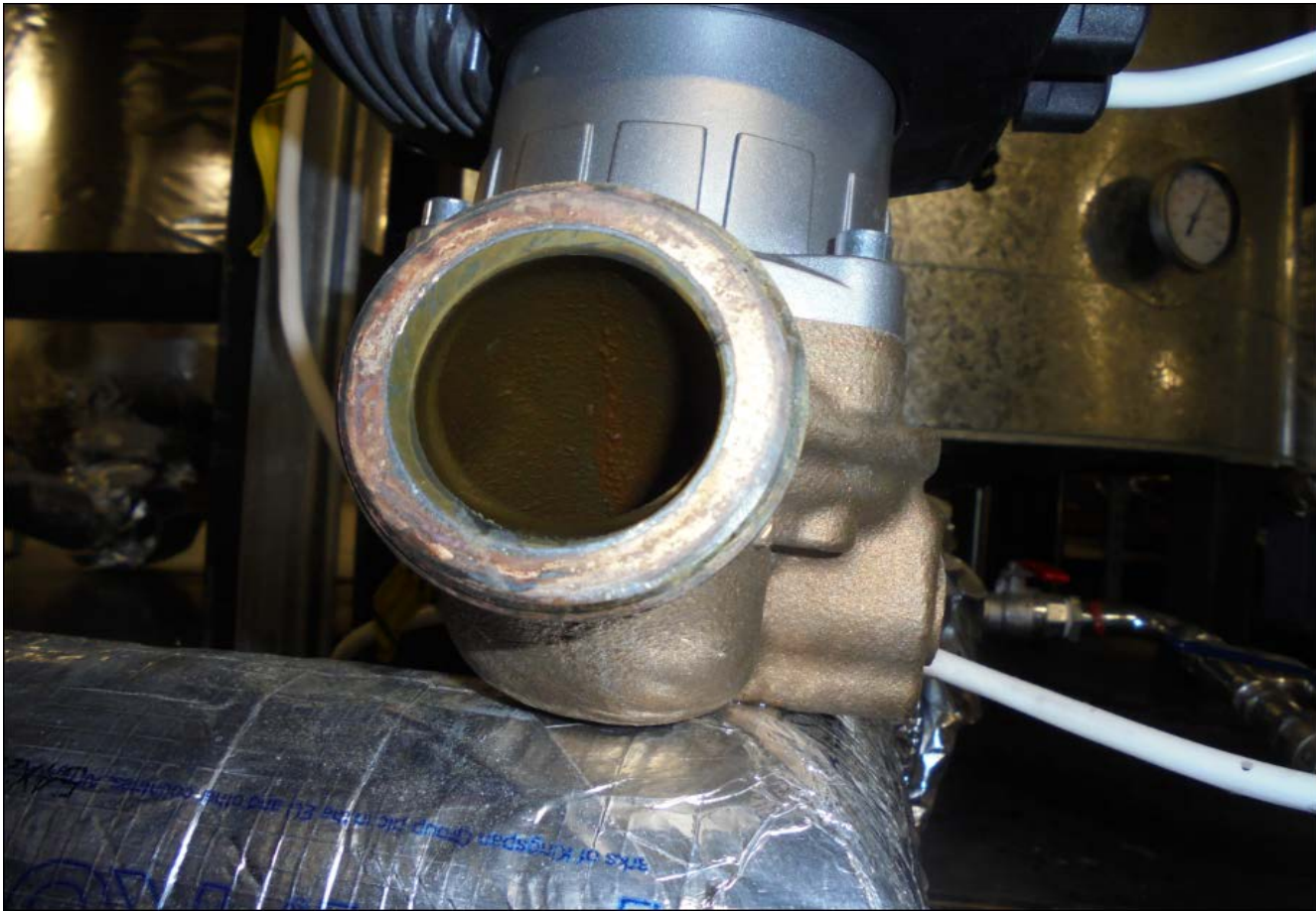
Fig 1 33Cal01 Shunt Pump
