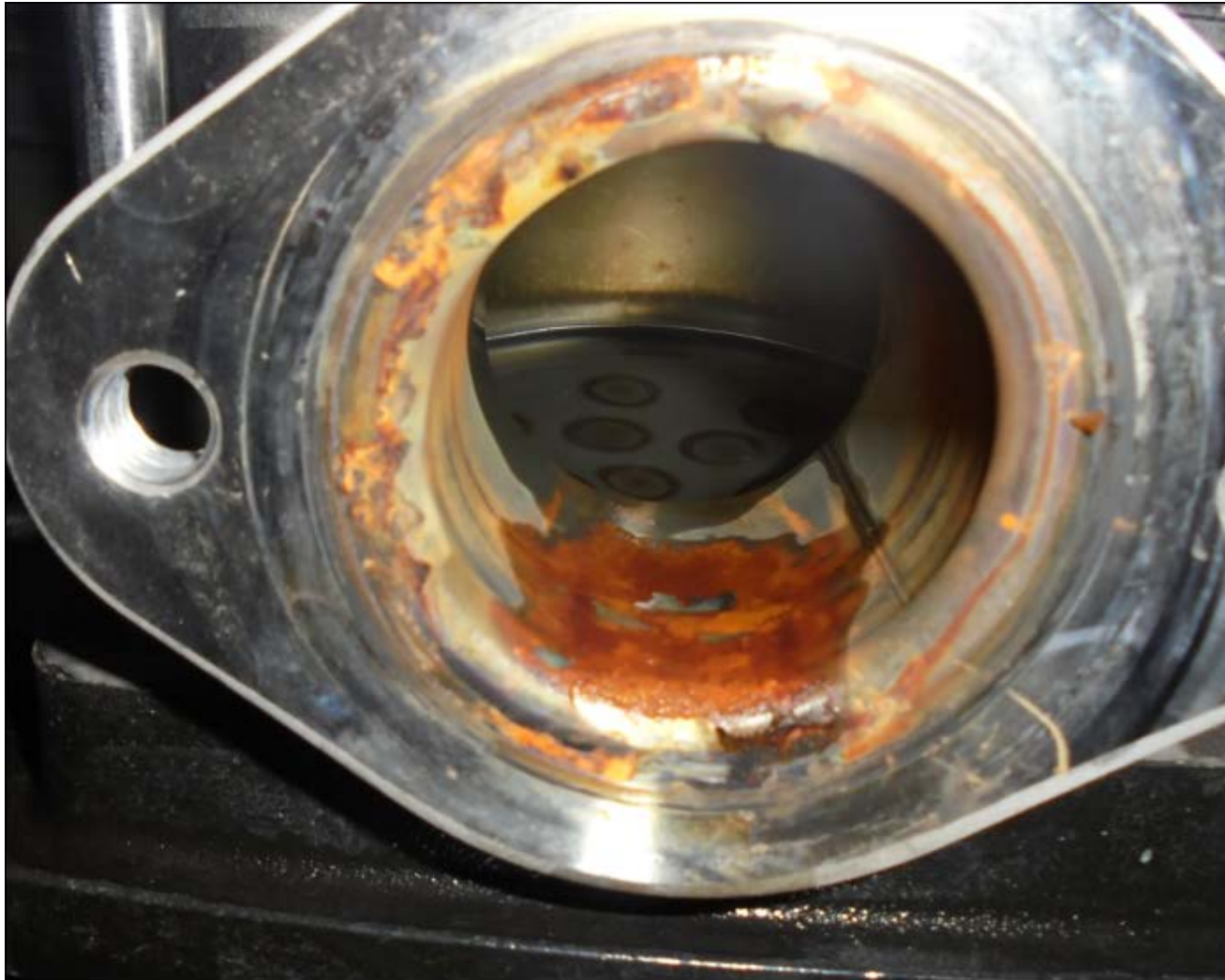
Fig 1 316, 1, 2 and 3 HWS Return Pump (internal)
