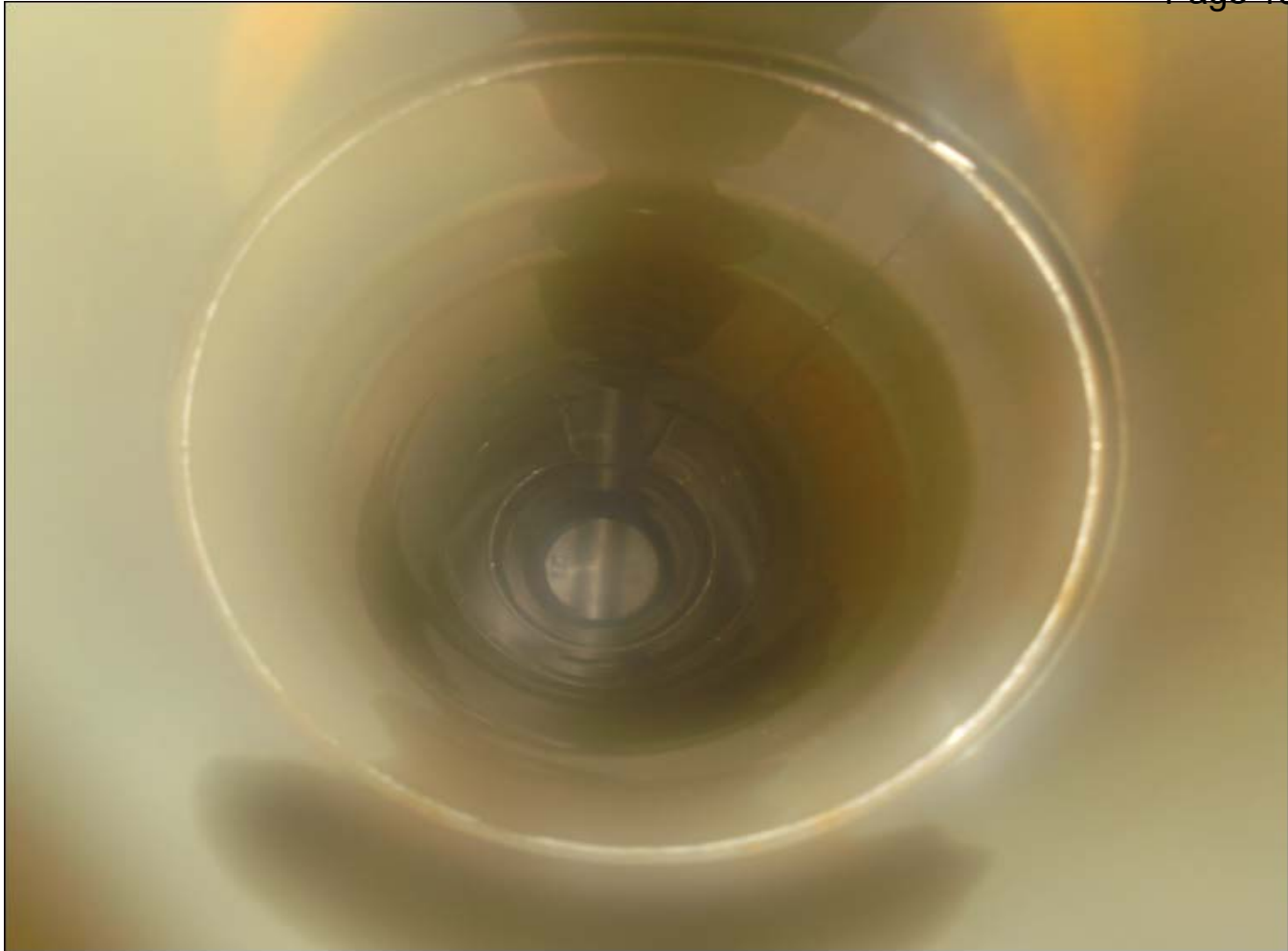
Fig 6 PR22 NRV HWS Return Line (SS Tube internal)
