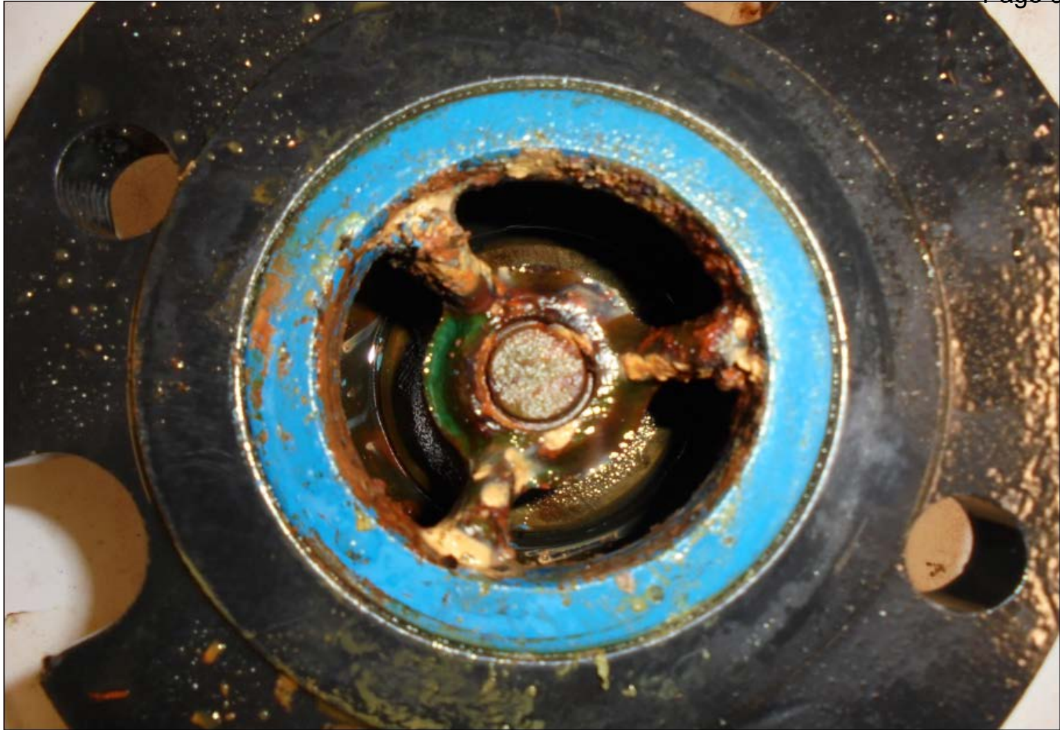
Fig 6 Booster Set 2 (Pump number 5 NRV) (Source NHS Scotland)
