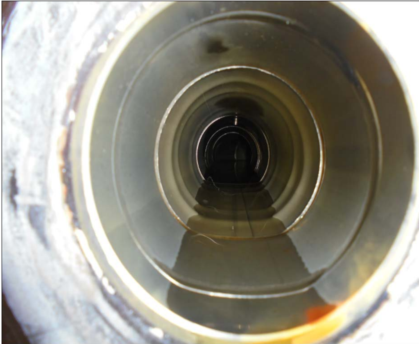
Fig 7 PR22 NRV HWS Return Line (SS Tube internal)
