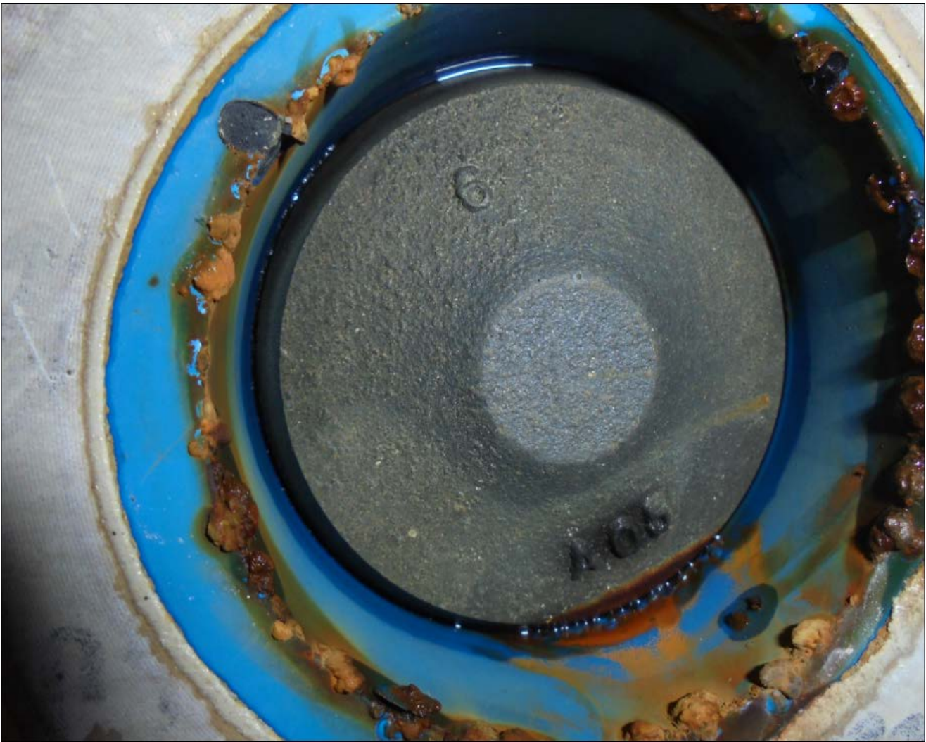
Fig 5 PR22 NRV HWS Return Line (internal)
