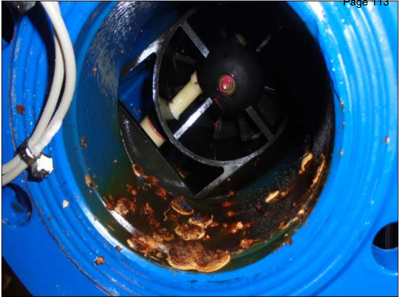
Fig 6 108mm CW Meter (internal)
