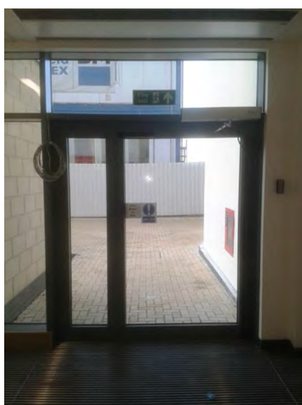
Push button not installed.
