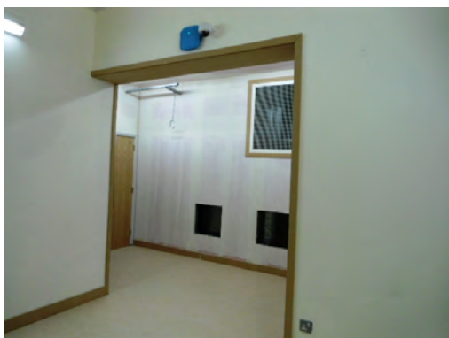
Some snagging work, painterwork and hatches required.
