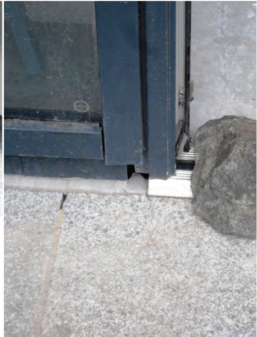
Excessive gap at the bottom of the door frame.
