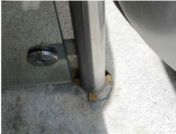
Timber wedges inappropriately used to support glazed panels.
