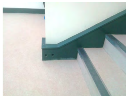
Holes to be filled in metal stringer.
