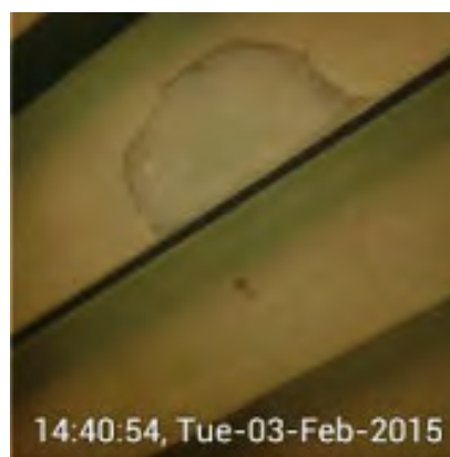
Damaged tread. There were other treads requiring repairs to lifting eyes.
