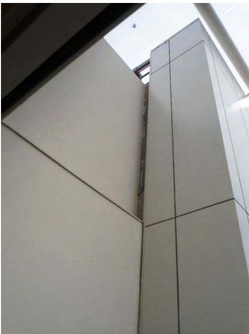
exposed concrete visible from Level 11 corridor.
