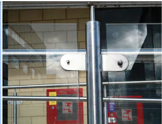
Nuts not fitted to glazed fixings to ramp.
