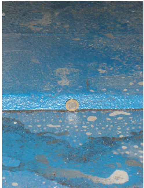
Level 3: Channel exceeds 30mm deep.
