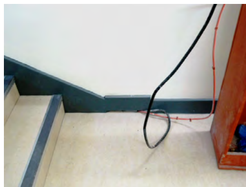
Site alarm system requires to be removed from some floors and skirting fitted.
