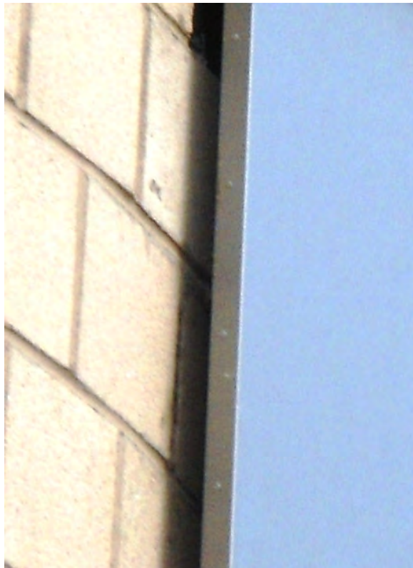
Gap between cladding and blockwork interface.
