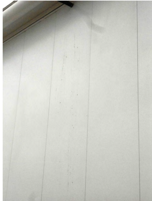
Pigeon droppings on cladding of Core B
