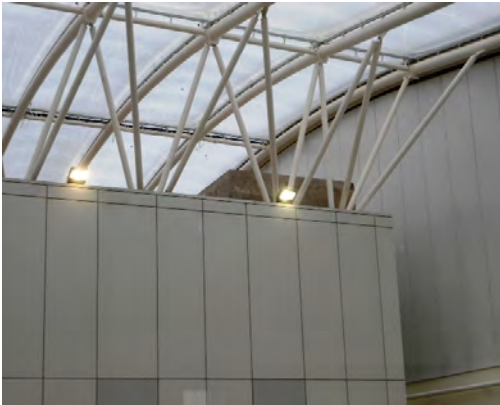
The concrete top of the lift enclosure in Core D is visible.
