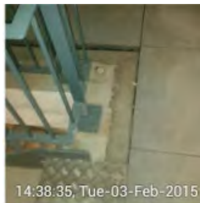
Edge of slab too high.
