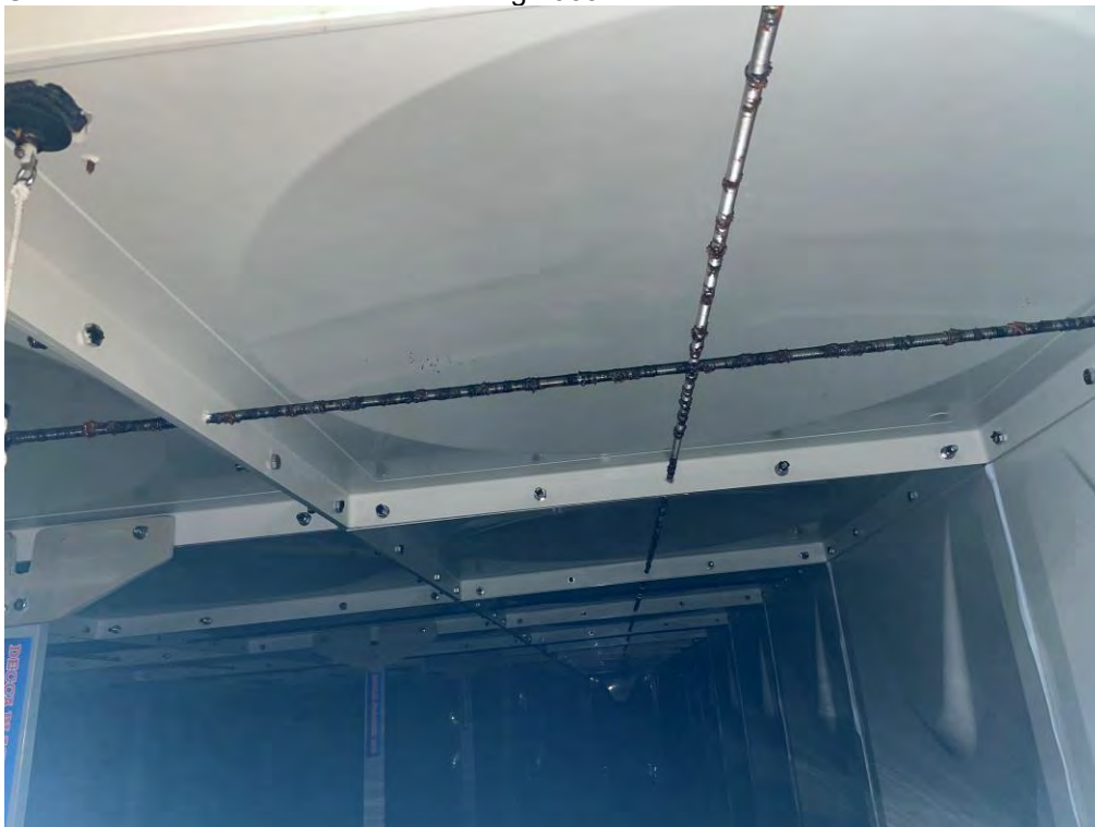
Corrosion of internal stainless steel image 005
