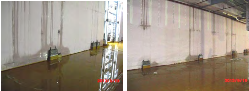
Water damaged boards.
