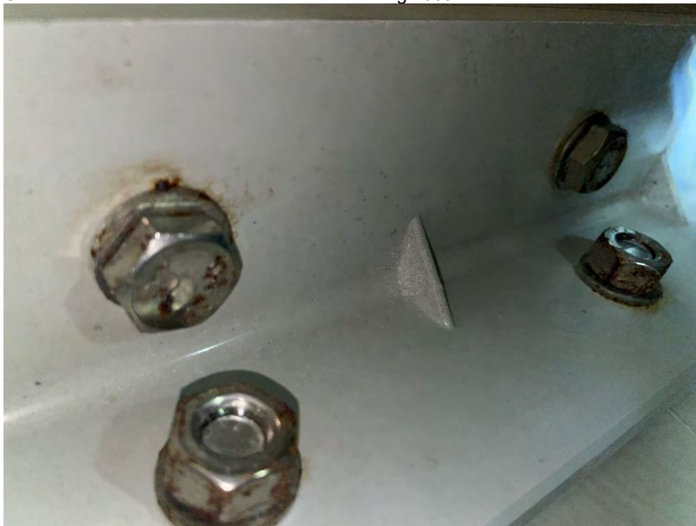
Corrosion of internal stainless steel fastener image 009
