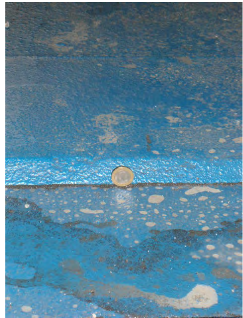
Level 3: Channel exceeds 30mm deep.
