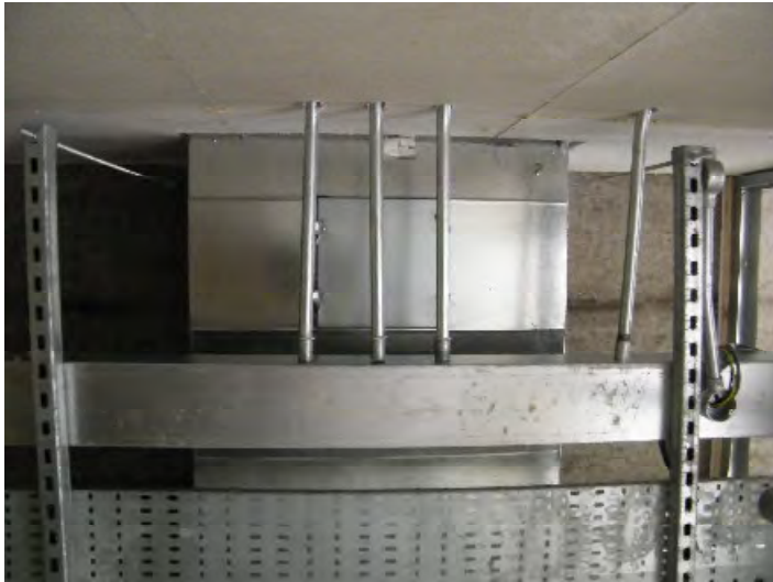
10. Typical Access Door Problem. March 2011.
