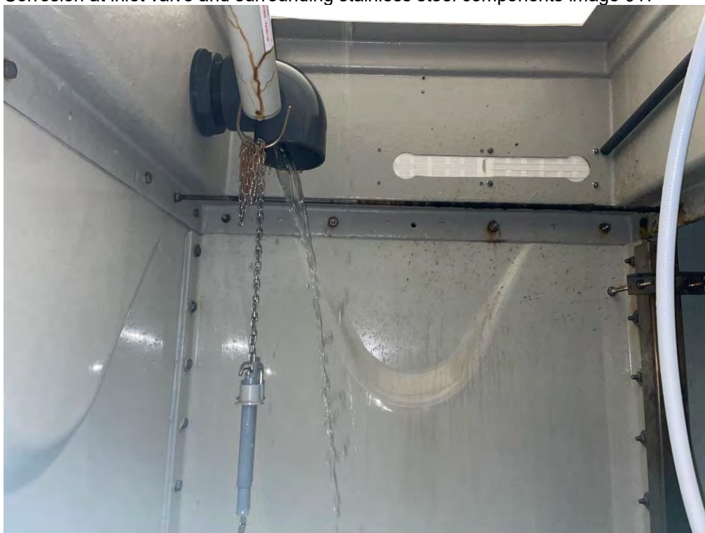
Corrosion at inlet valve and surrounding stainless steel components image 017
