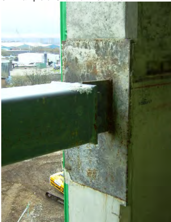
7. Rust on Steel Plate.
