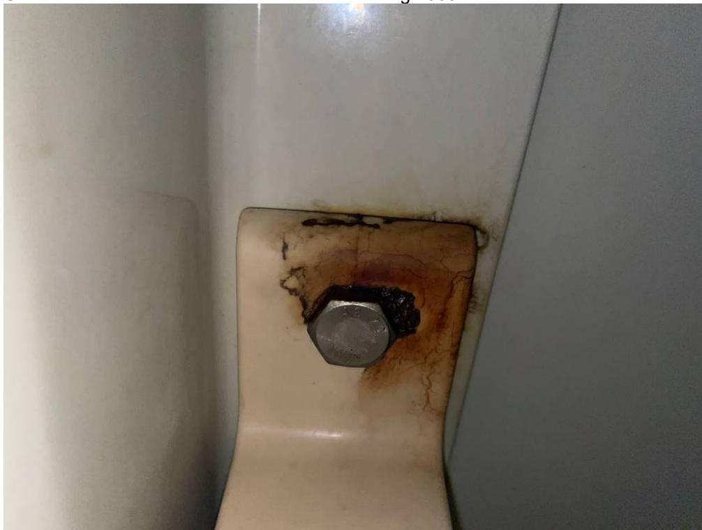
Corrosion of internal stainless steel fastener image 008
