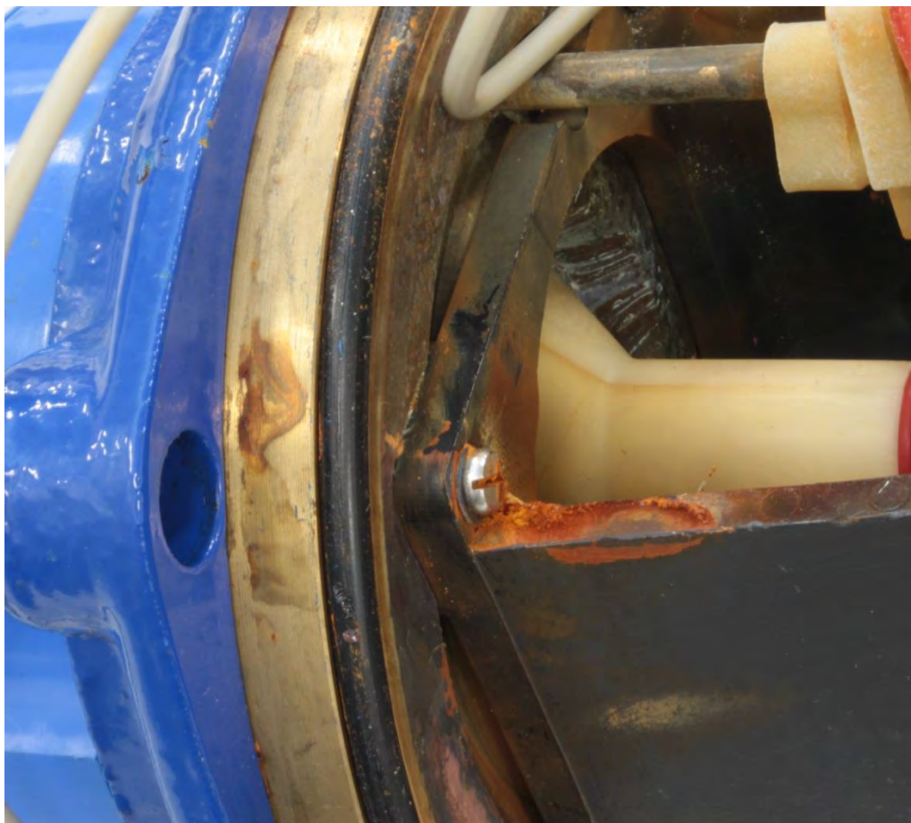
Figure 3: Transferred red/brown corrosion products with no evidence of corrosion on brass component.
