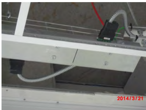
Room GENW 006 Cable plugged into Wago power outlet.
