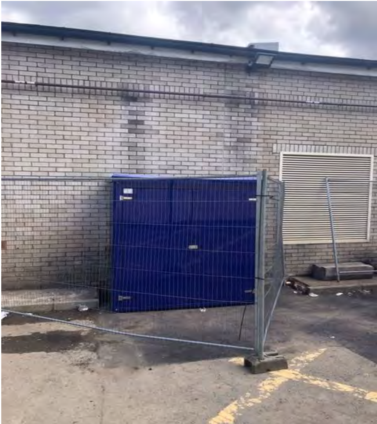
Installed in a kiosk
