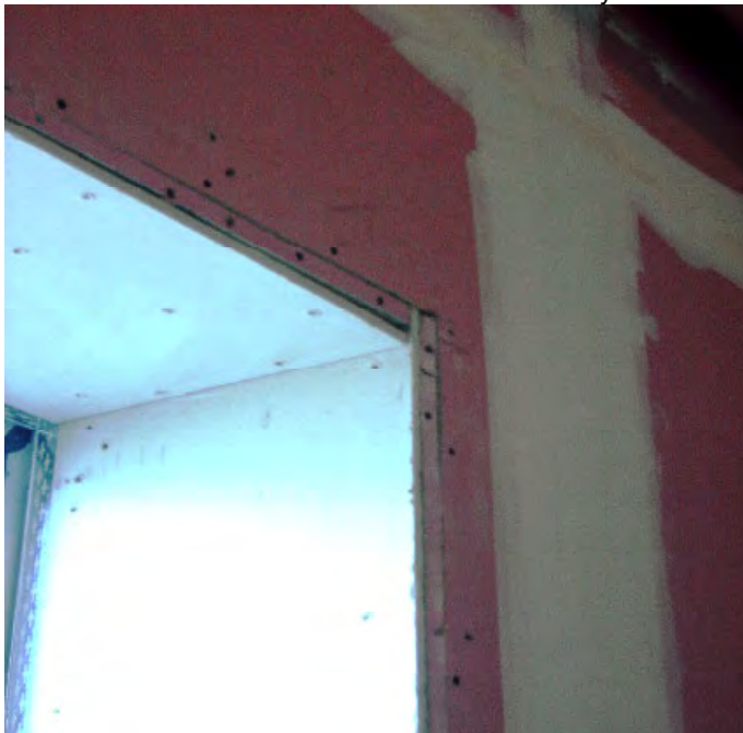
5. Insert pieces of boarding used as infills around the window reveals 23rd March 2011.
