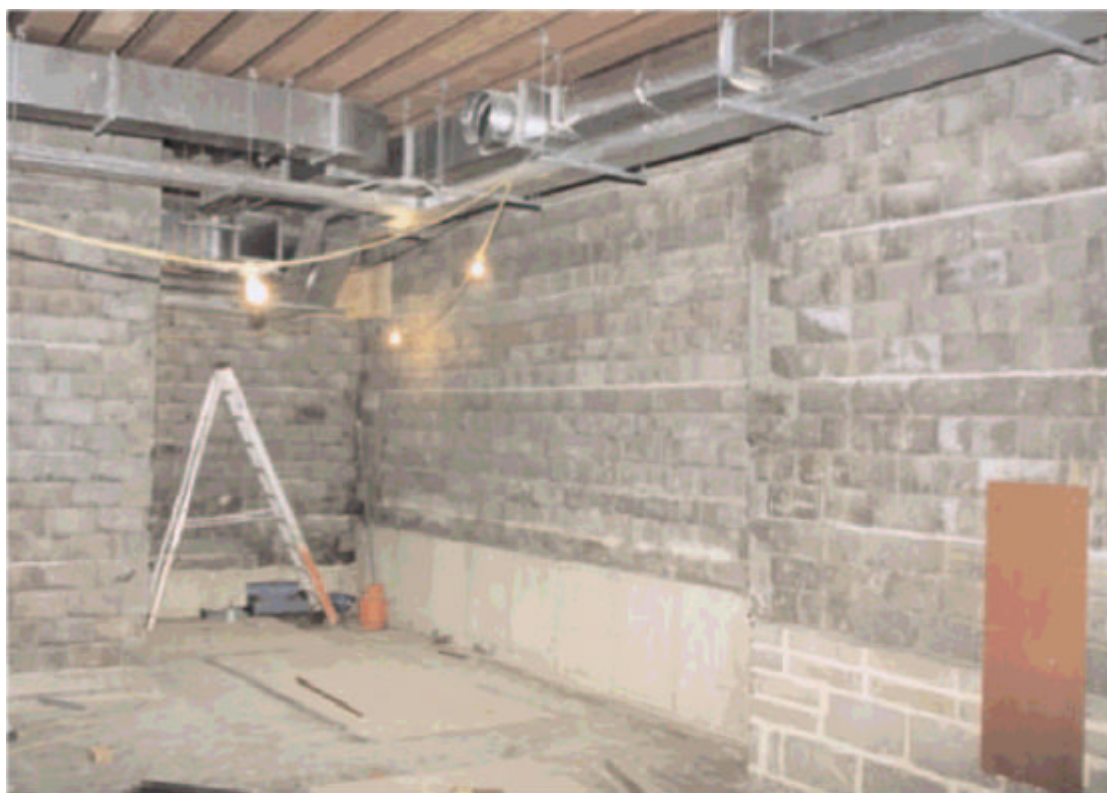
Internal view of linear accelerator bunker under construction using blocks of alternative shielding materials. Joints are formed using specialised proprietary mortar. Shows services entering from maze corridor and steel joists supporting roof structure.
