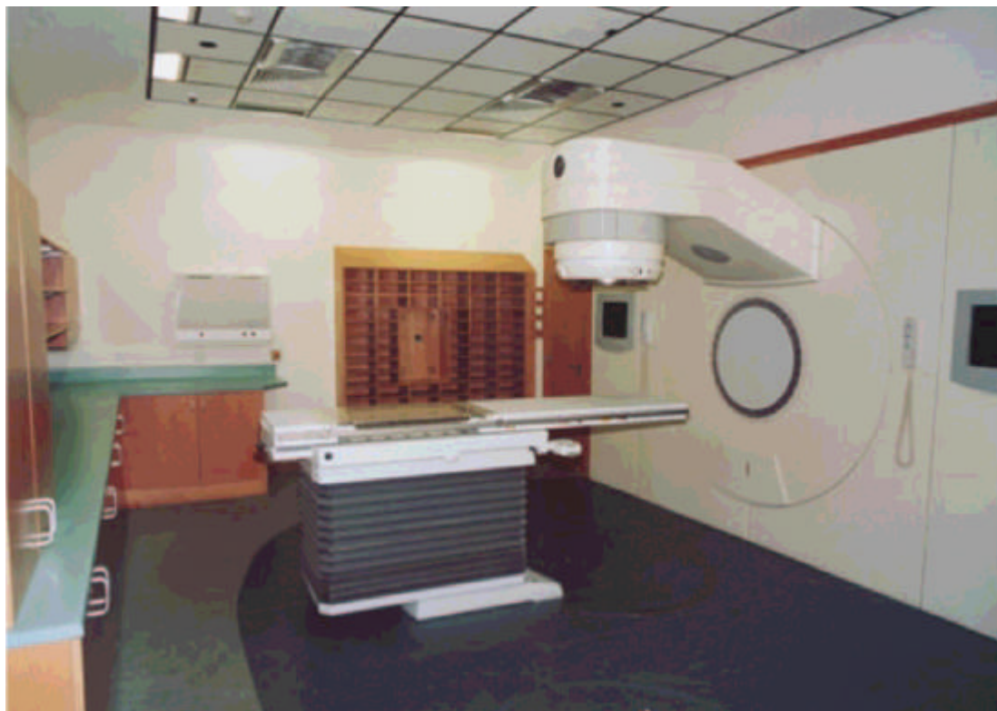
Linear accelerator treatment room where linac fascia panel is used to create a machine room
