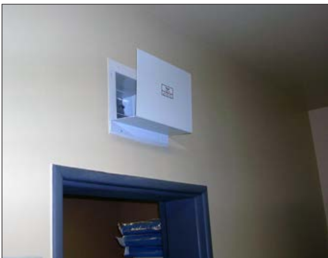
Pressure stabiliser fitted with stand-off baffle in preparation “lay up” room
