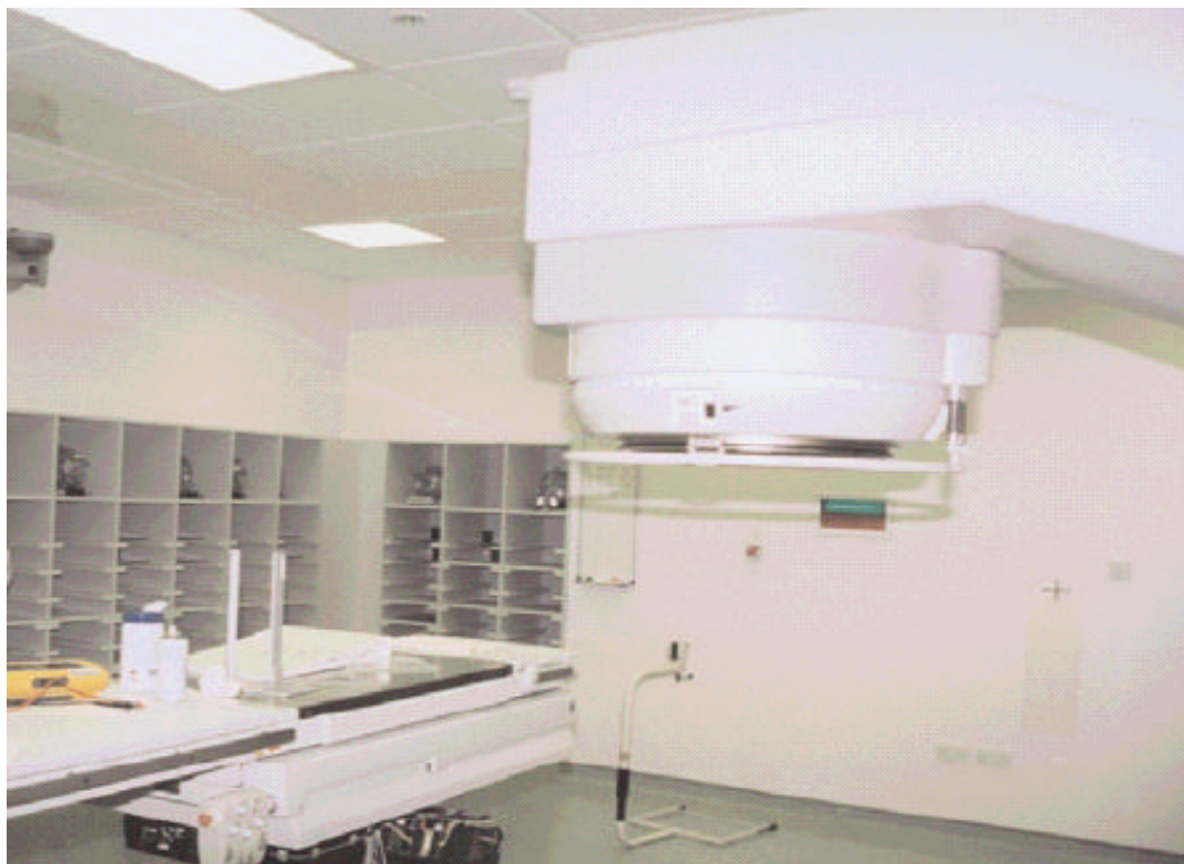
Linear accelerator treatment room showing customised storage facility
