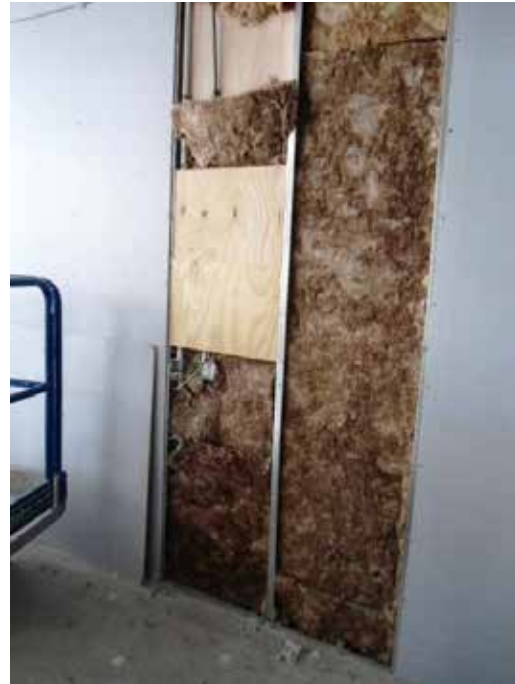
Room OPD1-077. Insulation missing Gaps between insulation at low level.
