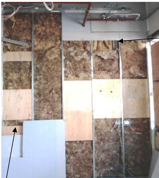
Insulation missing behind patress
