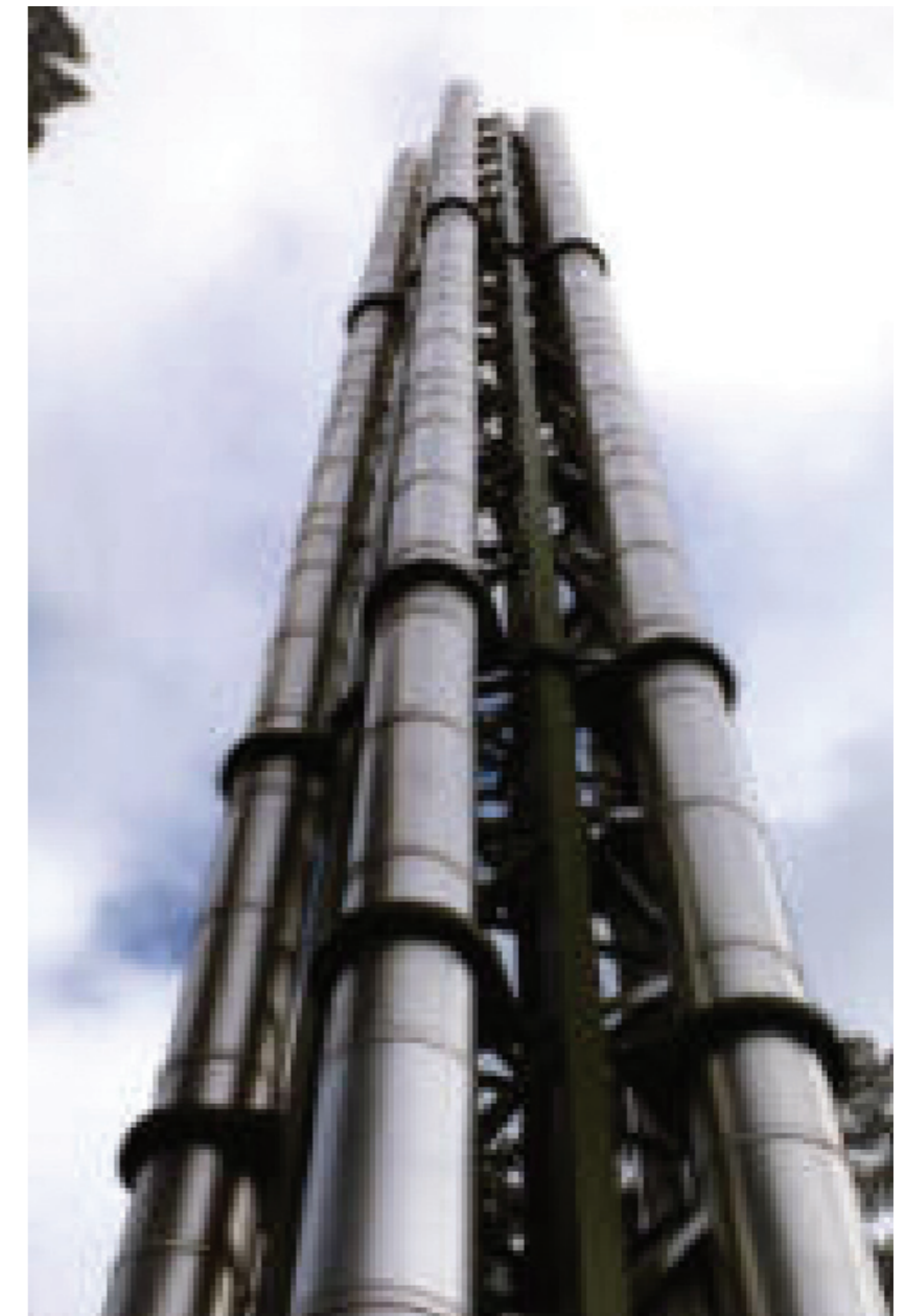
Multi core chimney
