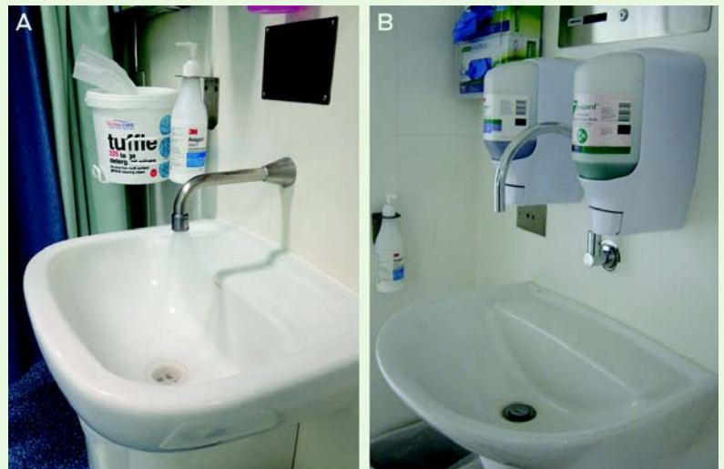
A: Existing sink, showing water spray directly over drain. B: Compliant sink design, showing larger basin and less forceful water flow directed away from drain, to prevent splash back and contamination with drain contents.
