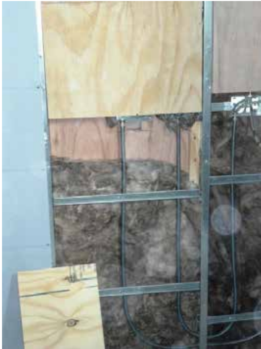
Room OPD1-101. Patress not fixed behind board and insulation missing.
