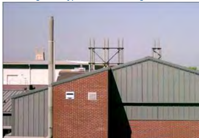
Figure 9 Typical LEV discharge stacks
