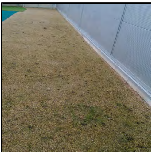
Fouling on astro turf
