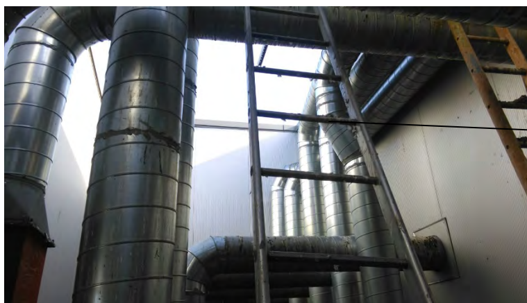
Pigeon fouling on plant room access ladders
