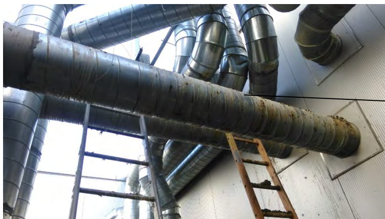
Ducting which has been heavily fouled.
