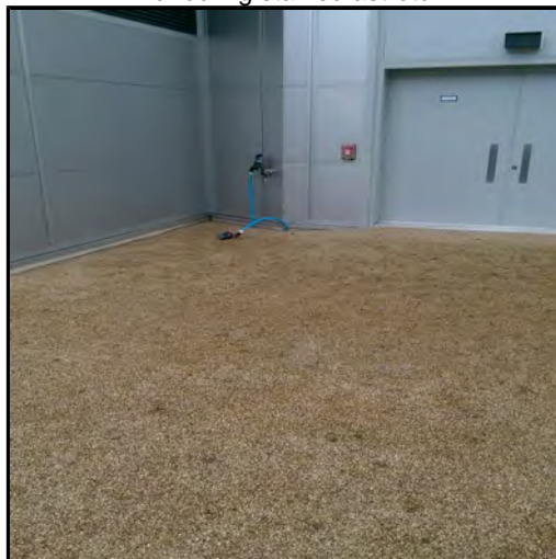
Fouling on sstro turf, tap nearby if useable will need a hose.
