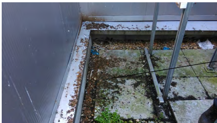
Fouled floor areas
