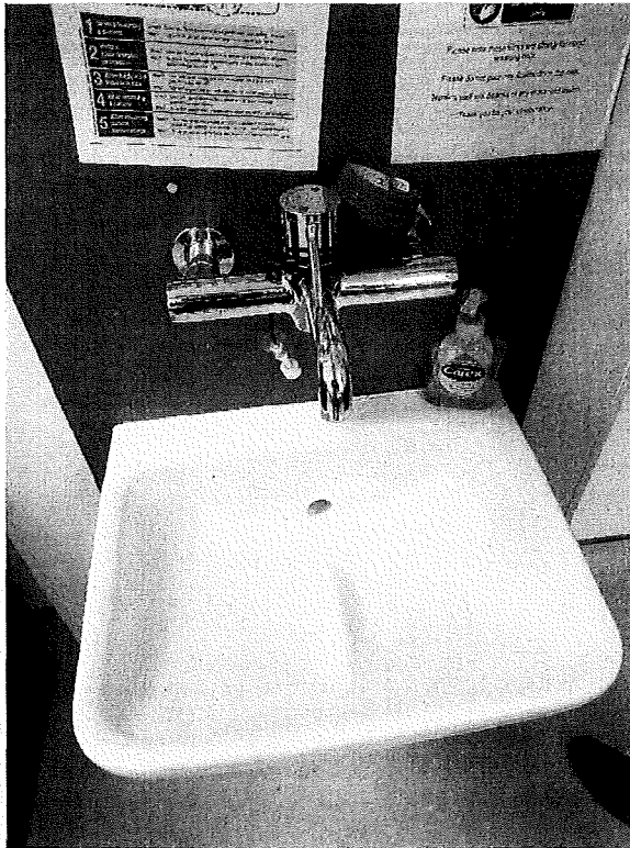
Photo 3. Photograph taken 2 nd December 2021: Ward 2B clinical consultants WHB. Auto flusher tied around monoblock tap head (unclear if this is a new or old auto-flusher), unclear if auto flusher is to be attached and suitable RAMS in place and reviewed. Also hand wash gel sitting on WHB bowl lip.
