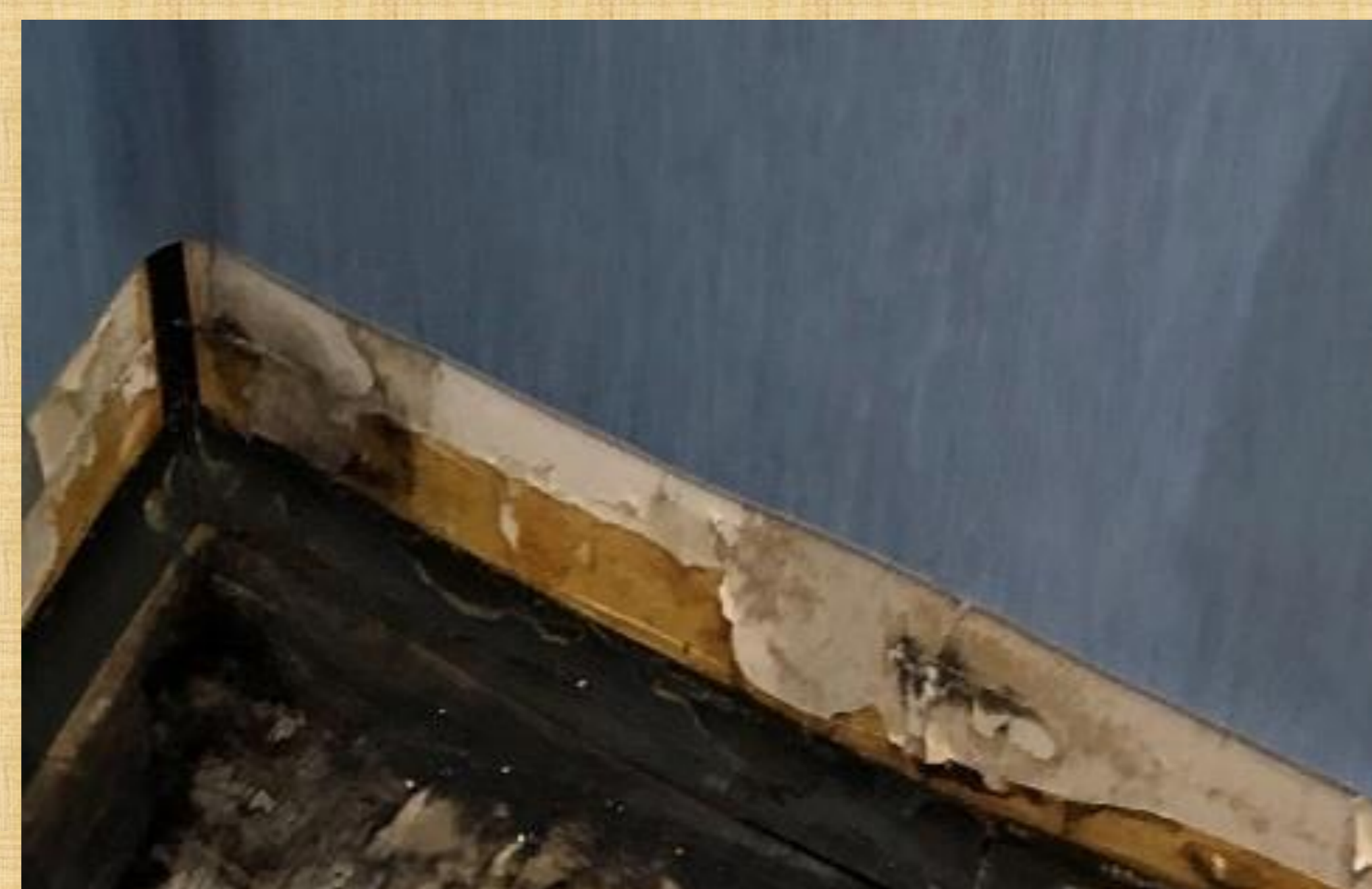
DAMAGED SHOWER FLOOR
