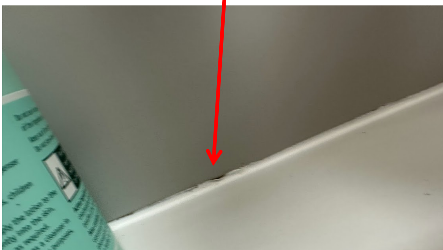
Figure 57. Sealant damage will result in moisture and biofilm retention
