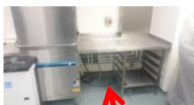
Flexible hoses on pressure reducing valves (assume to be EPDM)
