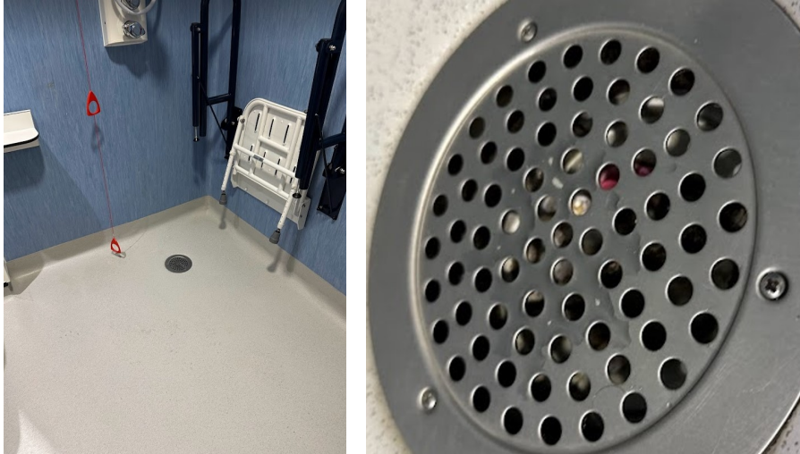
Figure 61. Staff reported poor drainage of showers and drain was visibly dirty.
