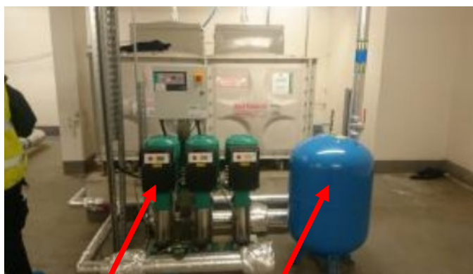
Trade booster pumps (green) with manifold and expansion vessels (blue)– source DMA L8 RA VT2.0
