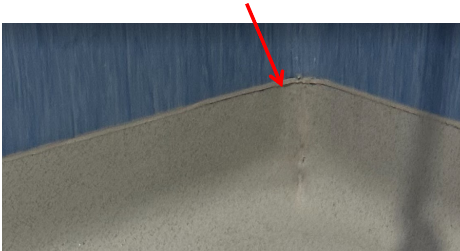
Figure 62. Gaps in sealant will retain moisture and drain related biofilm
