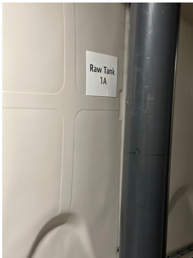
Figure 8. Raw water storage tank 1A.
