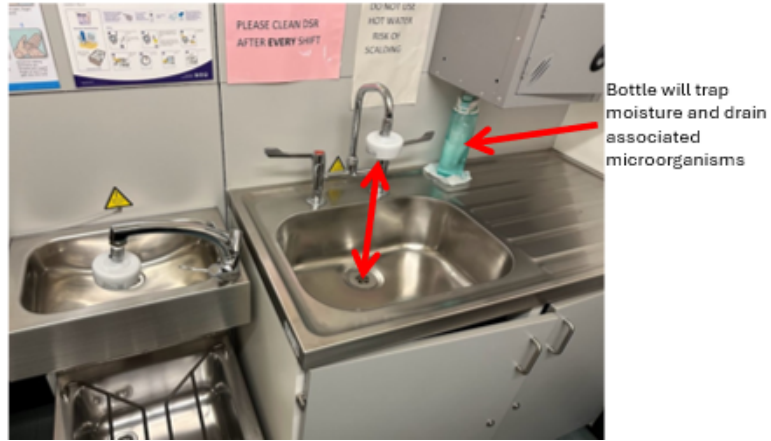
Figure 55. Excessive splashing of drain related microorganisms and inappropriate storage of items on sink.
