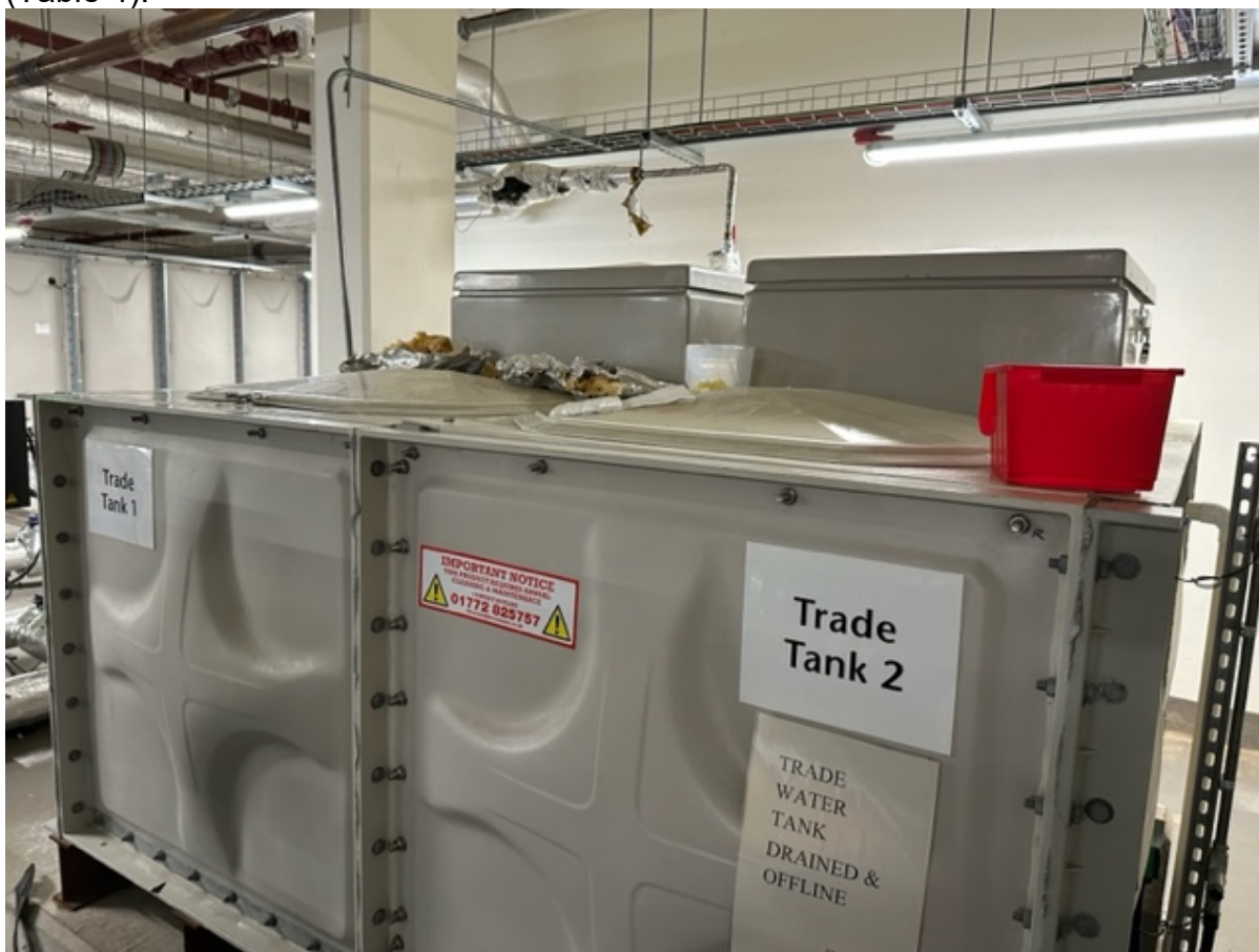
Figure 10. Trade water tanks
