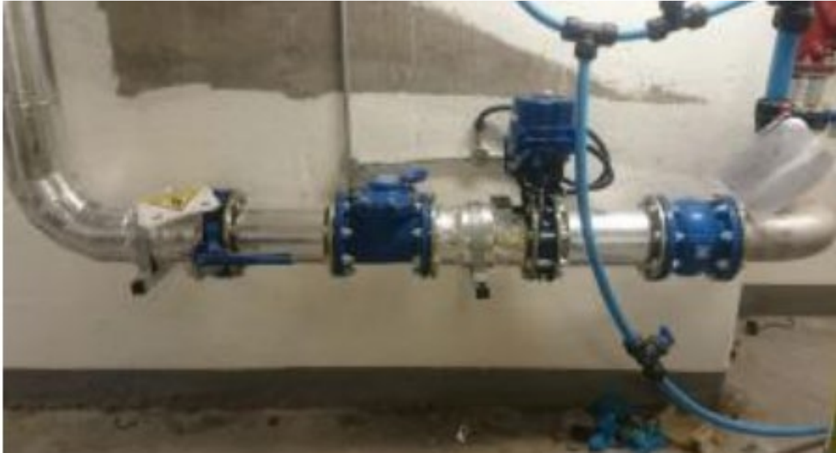
Figure 4. Hardgate mains water supply Image 93 .
