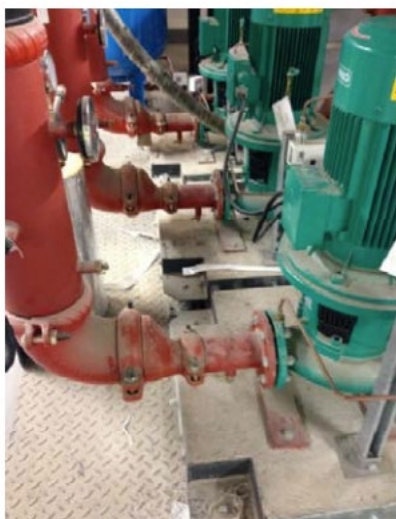
Figure 33: Low Temperature Hot Water (LTHW) pumps 150
