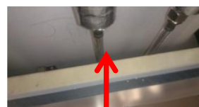
EPDM flexible hoses fitted at double level sinks in facilities room (DSR's)
