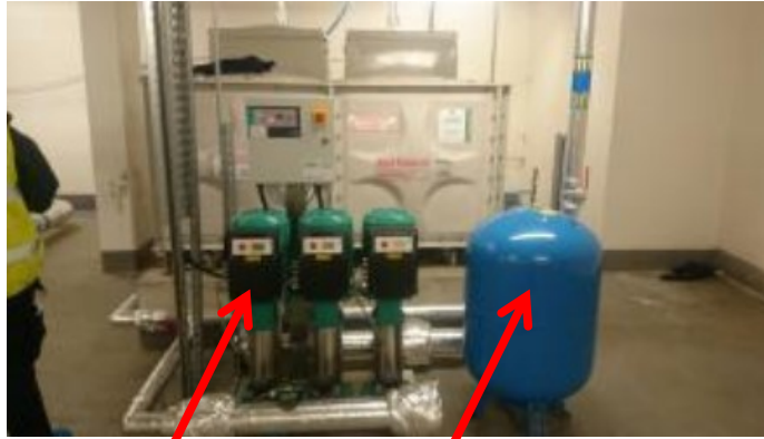
Trade booster pumps (green) with manifold and expansion vessels (blue)– source DMA L8 RA VT2.0
