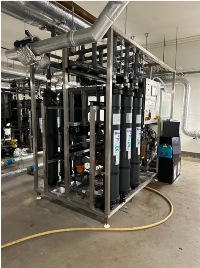
Figure 11. Elga ultrafiltration unit
