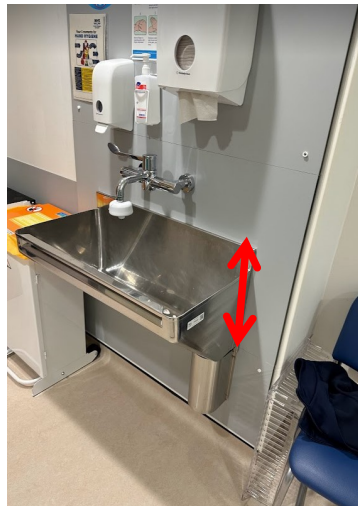
Figure 54. Excess splashing due to deep trough sink
