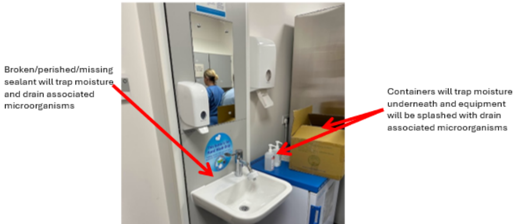
Figure 53. Inappropriate storage of materials within the splash zone of the sink
