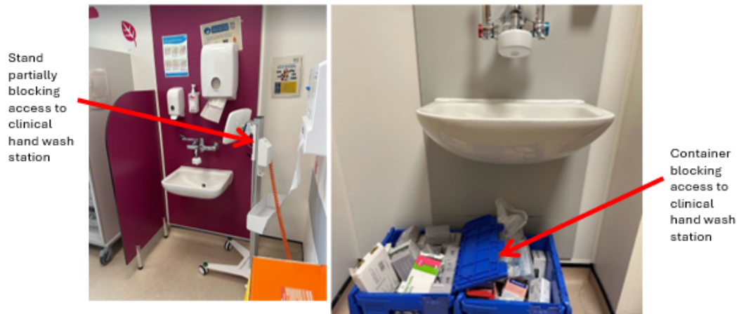
Figure 49. Storage of equipment and boxes that i) will prevent access to sinks and ii) will be splashed by contaminated water from the sink
