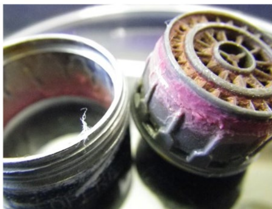
Biofilms on outlet fittings
