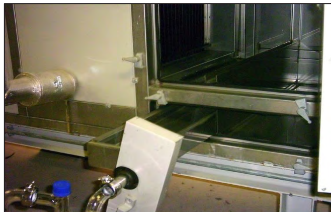
Figure 7 Removable AHU drainage tray
