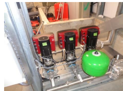
Boosted Pump Set
