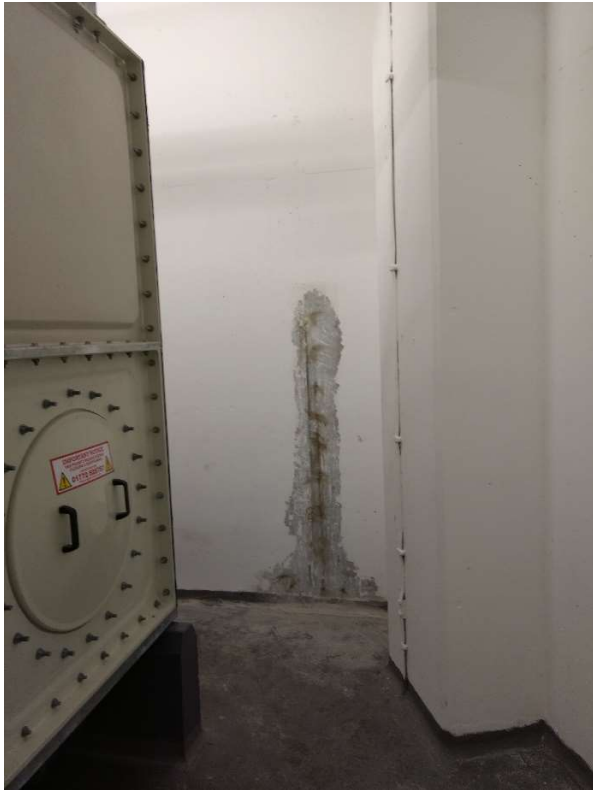
3 – Evidence of damp proofing requiring QA
