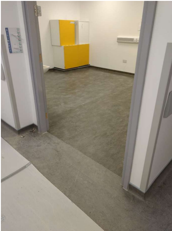
1 – Very noticeable batch variations between rooms – Dental room
