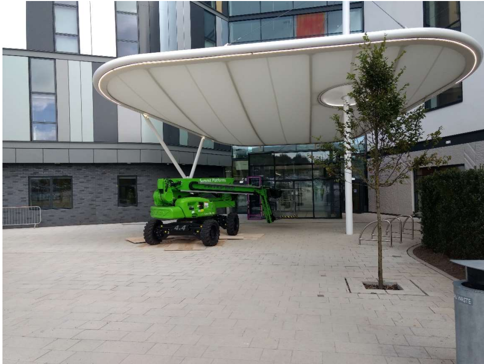
7 – Heavy machinery operating on paved areas without adequate weight spreaders
